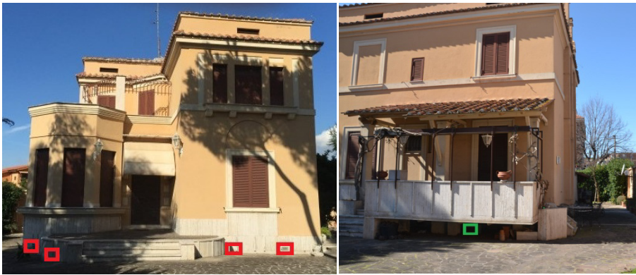
Figure 2: Left: the residential building main facade; windows for the basement ventilation are highlighted in red boxes. Right: building eastern facade; the venting hole from the cellar is highlighted in the green box.
