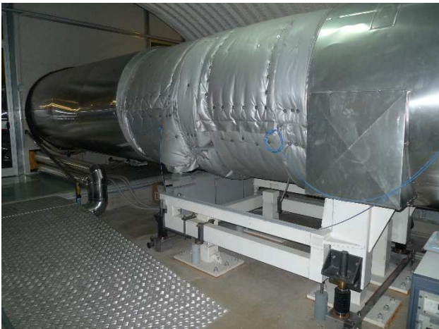
Figure 3: End Building-Tunnel link module. Special tube support with micrometric mechanical realignment system.
