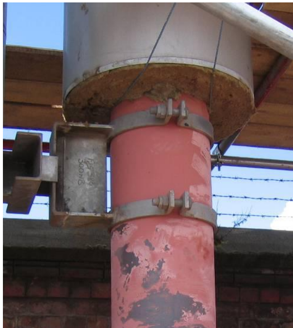
Figure 7.3: Picture of clamp used to hold steam line in place at Port of Liverpool power station.
