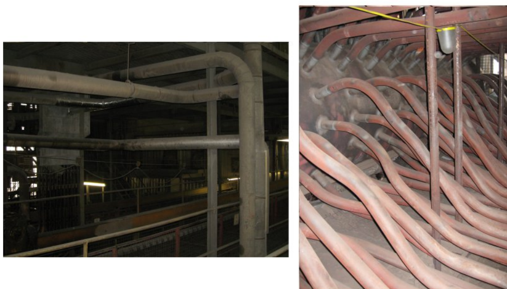
Figure 1.4: Some examples of pipework found in a power station.
