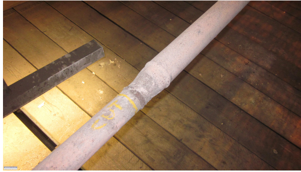
Figure 6.3: Photograph showing reducer connecting 2 inch supply to sootblower B29 with 2.5 inch main supply pipework
