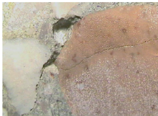
Fig. 18 Cracks around the perimeter of aggregates and inside the reddish aggregate (sample label: Beam 3).
