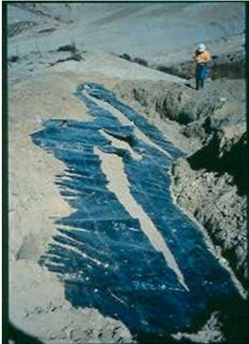
Figure 1-1: Geomembrane tear at Cell C, Chiquita Canyon Landfill following the 1994 Northridge earthquake
