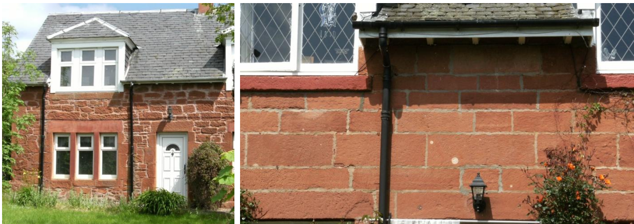
Fig. 19: Wester Cottage at Ballindean. Early 19 th century build with squared and coursed fine grained orange/red sandstone walling and dressings. The orange/red sandstone of the 19 th century cottages has extremely characteristic reduction spots. None of which was found in the sandstone of Westown Kirk.
