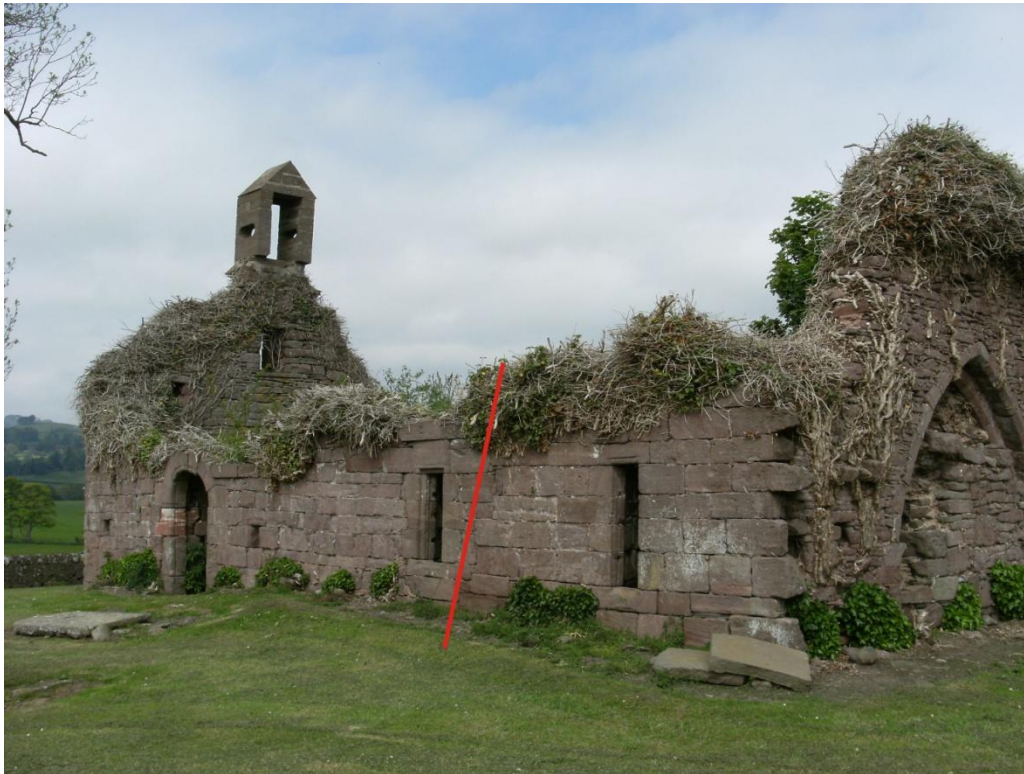
Fig. 6: South elevation showing discontinuity in the masonry between the eastern section and the rest of the building (highlighted by vertical line).
