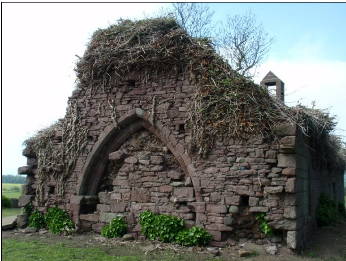
Fig. 3: Eastern gable wall with pointed chancel-arch. The infilled wall probably represents the post-reformation alterations making the building a ‘suitable preaching station’.
