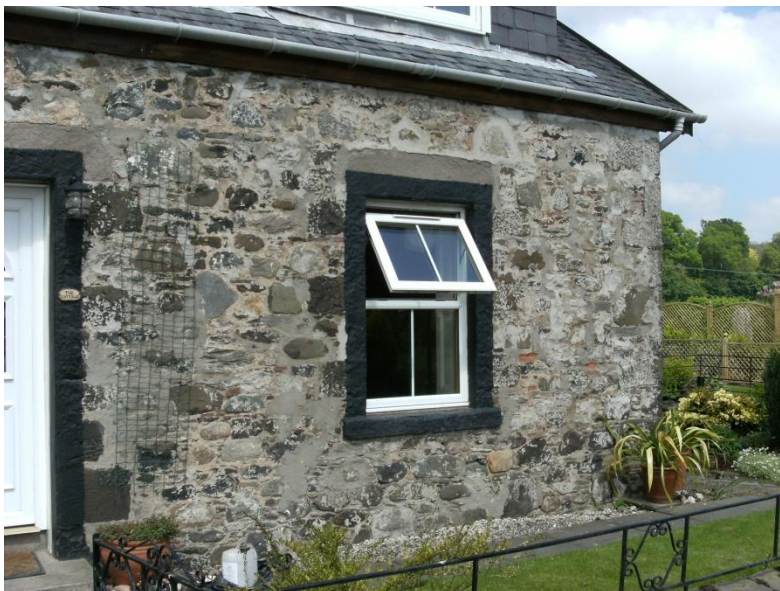
Fig. 16: Traditional cottage in the nearby village of Rait, constructed of random rubble comprising mixed purple sandstones and whinstone boulders, with dressings of purple flagstone (mostly overpainted).
