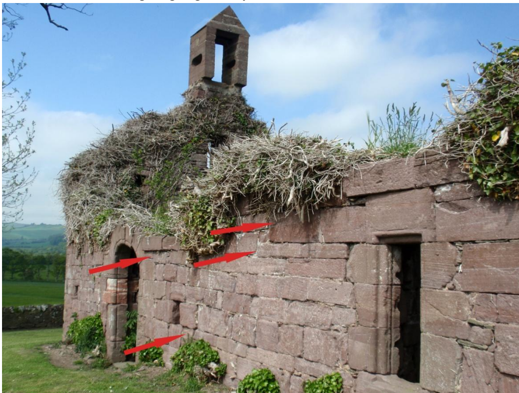
Fig. 7: Detail of south elevation showing 'wedging out' of masonry courses along the wall from east to west (highlighted by arrows).
