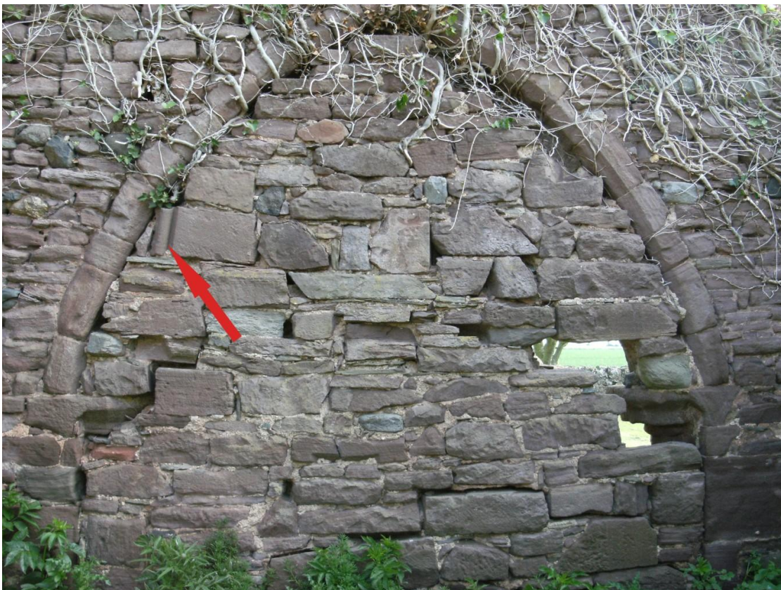
Fig. 9: Arch infill on the east gable containing reused masonry block with moulded detail (arrowed).
