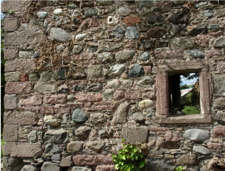
Fig. 17: Rait Old Parish Church contemporary to Westown Kirk. Random rubble walling with significantly smaller block sizes and masonry styles than found at Westown Kirk as illustrated in quoins (left) and the window surrounds.
