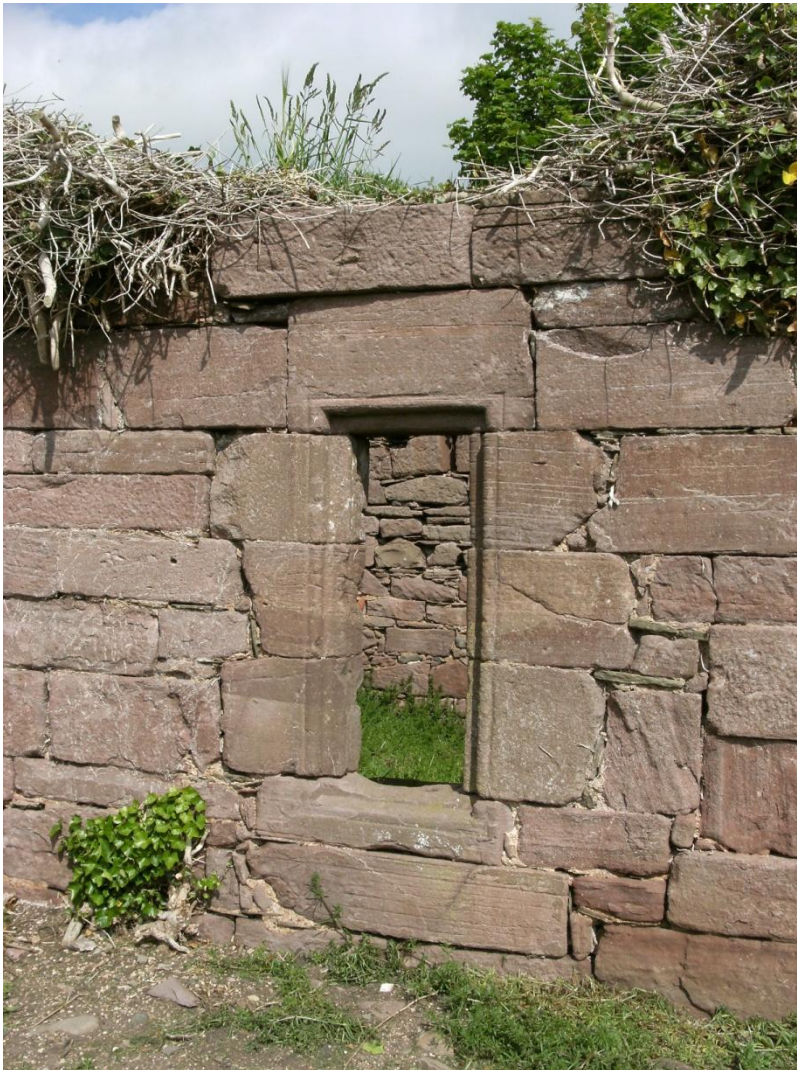
Fig. 8: Window on south elevation with lintel block of greater height than adjacent blocks in the same course, suggesting that the lintel stones may not be the original blocks for the windows.
