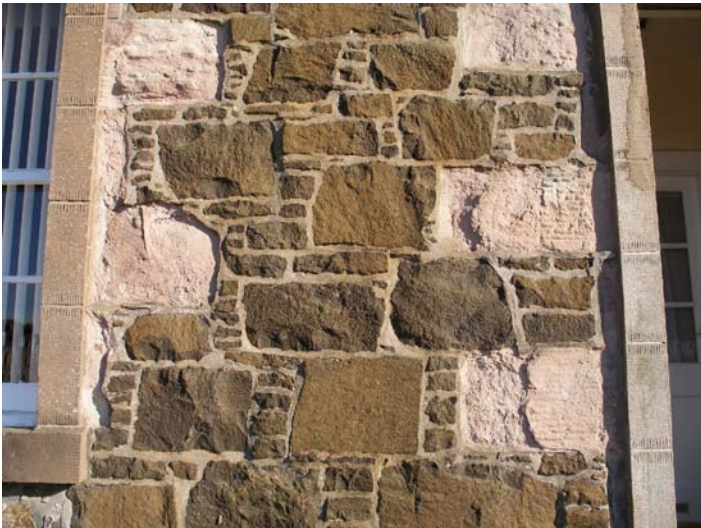
Fig. 7. Detail from above showing the Rothesay greenstone (weathering to dark brown) comprising roughly squared large block and smaller 'sneck' stones giving a highly distinctive masonry style. The pale sandstone dressings are undergoing severe stone decay with surface loss.
