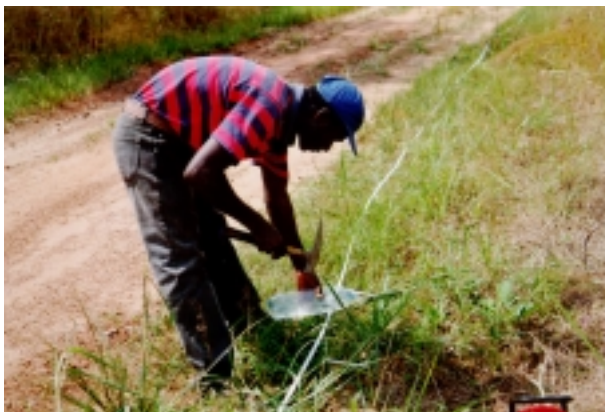
Plate 11. Electrodes being watered to ensure good contact with the ground for a resistivity survey.
