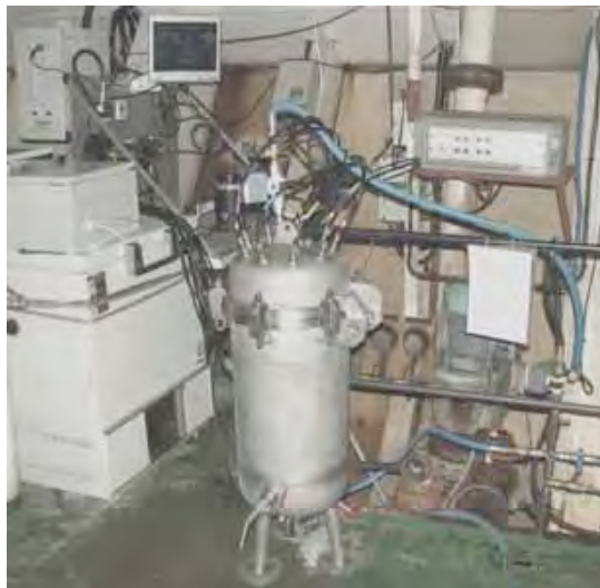
SNOMS OceanBox tank and electronic cabinet in the forward pump room of the P&O Pride of Bilbao 23 November 2006
