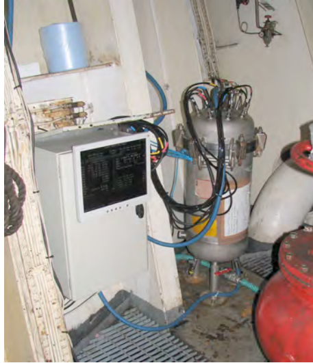
The SNOMS tank and electronics box in the machinery space on the Pacific Celebes
