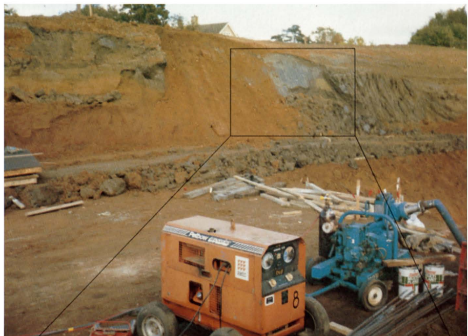
Plate 4 Cutting in Gault clay on the route of the M40 Motorway where a slide has occurred on a discontinuity in the clay which is dipping out of the cut face at a high angle. The face is capped by a thin layer of gravelly sand.
