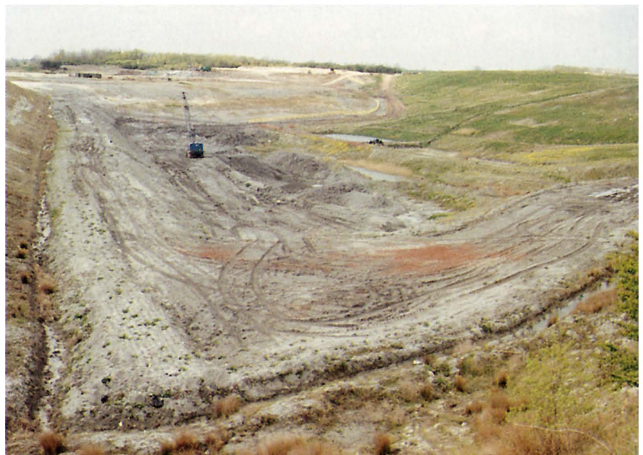
Plate 5 Arlesey Brickpit. Remoulded, wet Gault clay in the pit floor causing poor trafficability.
