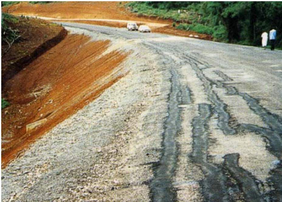
Figure 1. Cracking in a red soil road embankment in Kenya. Cracks up to six centimetres wide have been repaired with asphalt [10]
