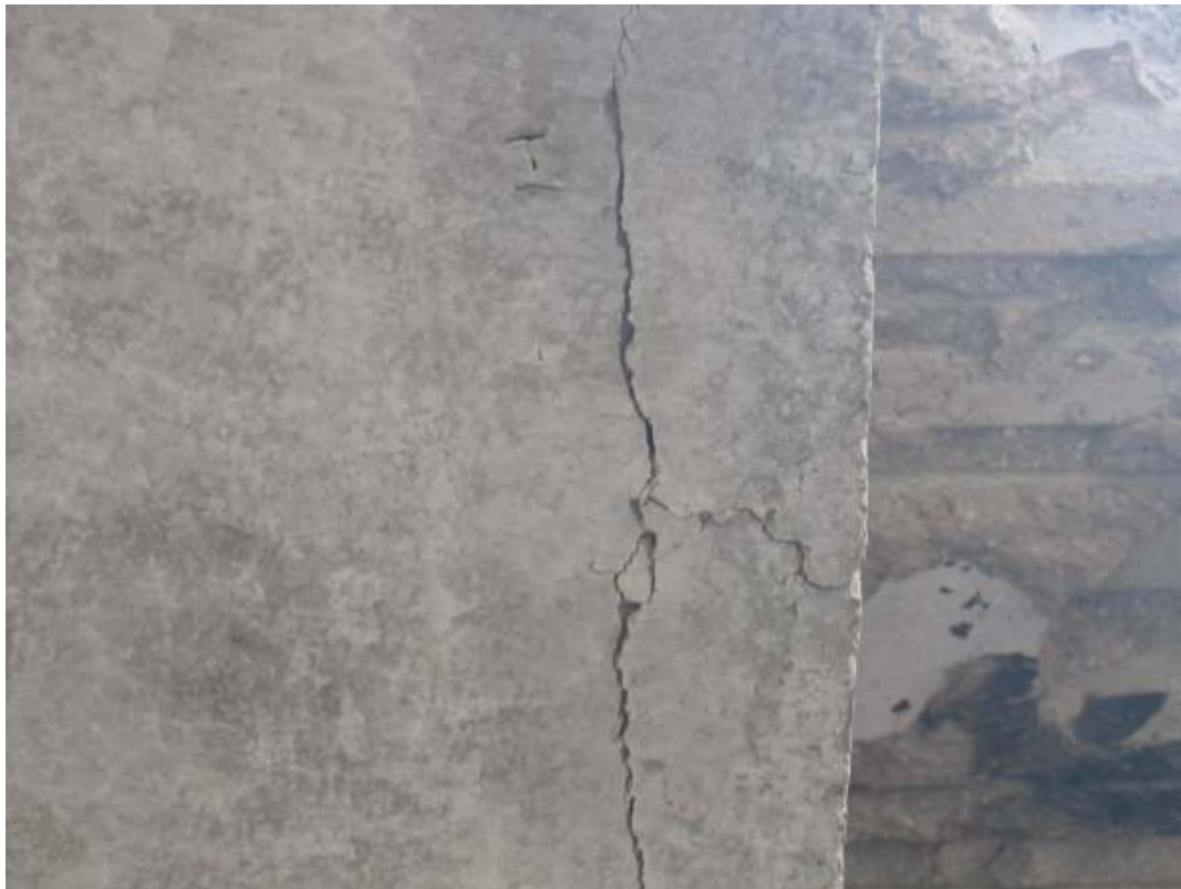
Figure 6 Cracks in a reinforced concrete column
