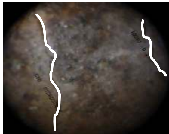
Figure 8 Shrinkage cracking occurrence on plain concrete
