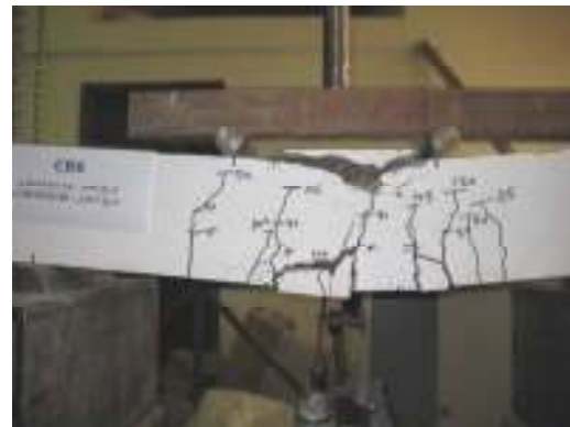
Figure 17 mode of failure CB6
