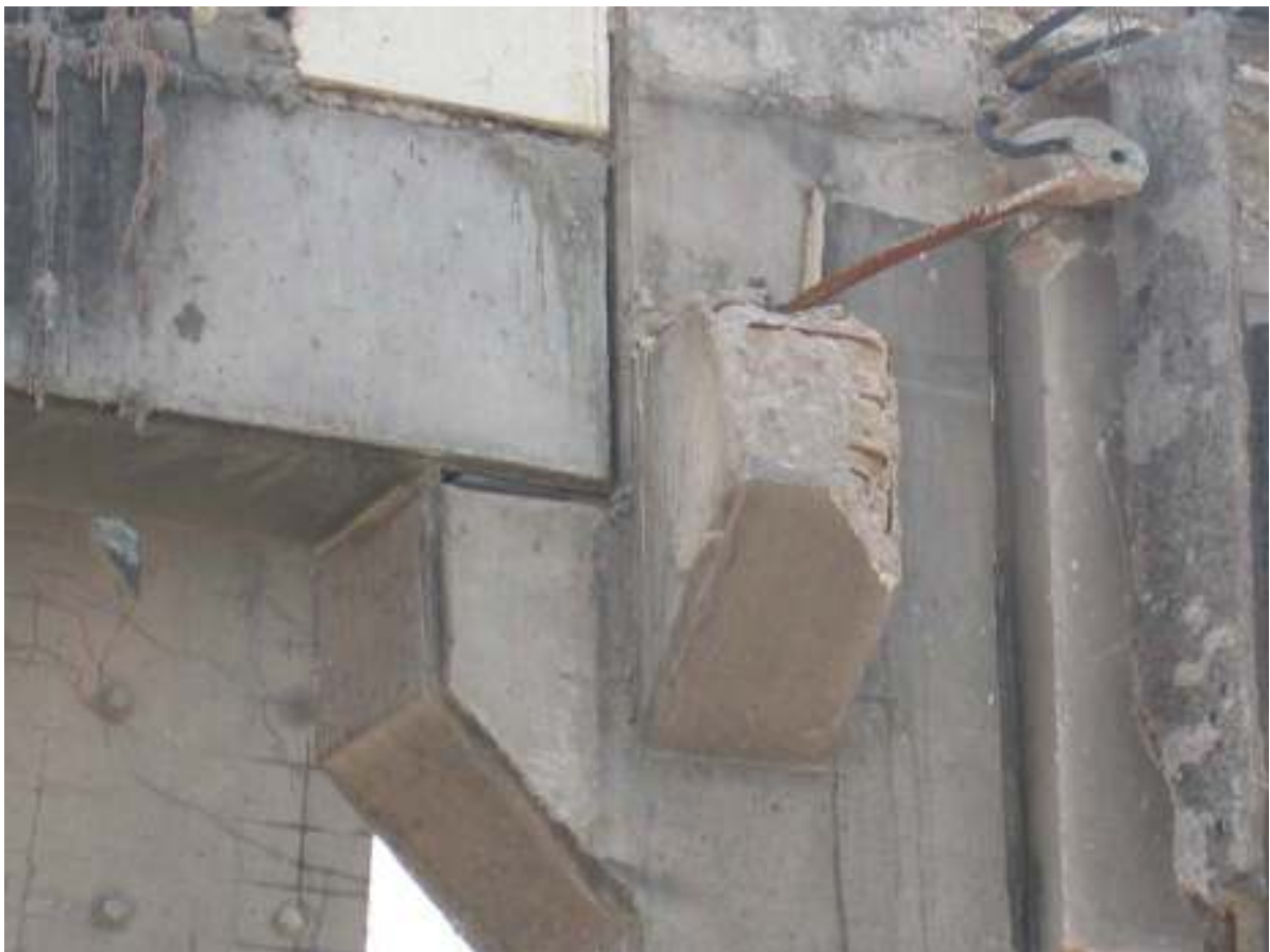
Figure 3 Cracks in column and spalling of corbel concrete
