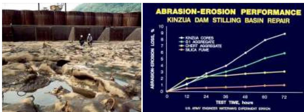
Figure 2 Kinzua Dam: The damage shown is in 1983, after only 9 years. The repair concrete using silica fume (lowest abrasion result in the USAEWES test) is not even being considered for replacement (2012).
