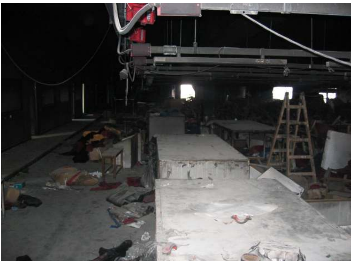
Figure 5 Post fire inside view of the 1st floor within Zone 3
