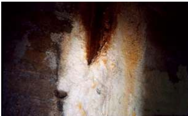
Figure 4 Calcite deposits on the wall of the inspection gallery
