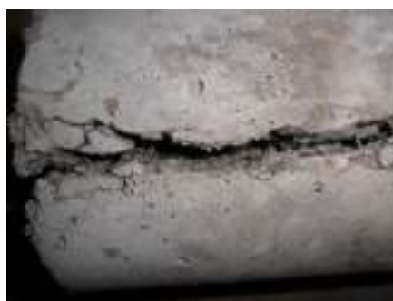
Figure 13 Type of failure
