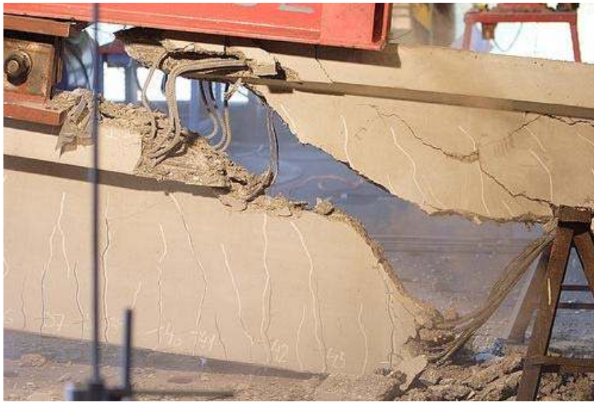
Figure 4 Breaking of beam F.P.02
