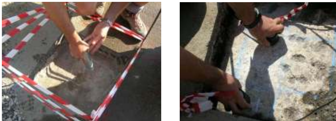
Figure 2 a) Schmidt rebound hammer test, b) Ultrasonic pulse velocity test on bridge slab
