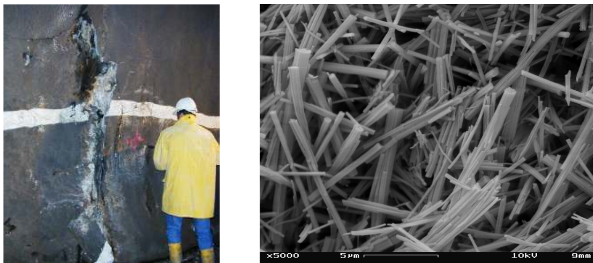
Figure 1 Concrete destroyed by thaumasite formation (left) and secondary electron image (SEI) of thaumasite crystals in deteriorated concrete (right)
