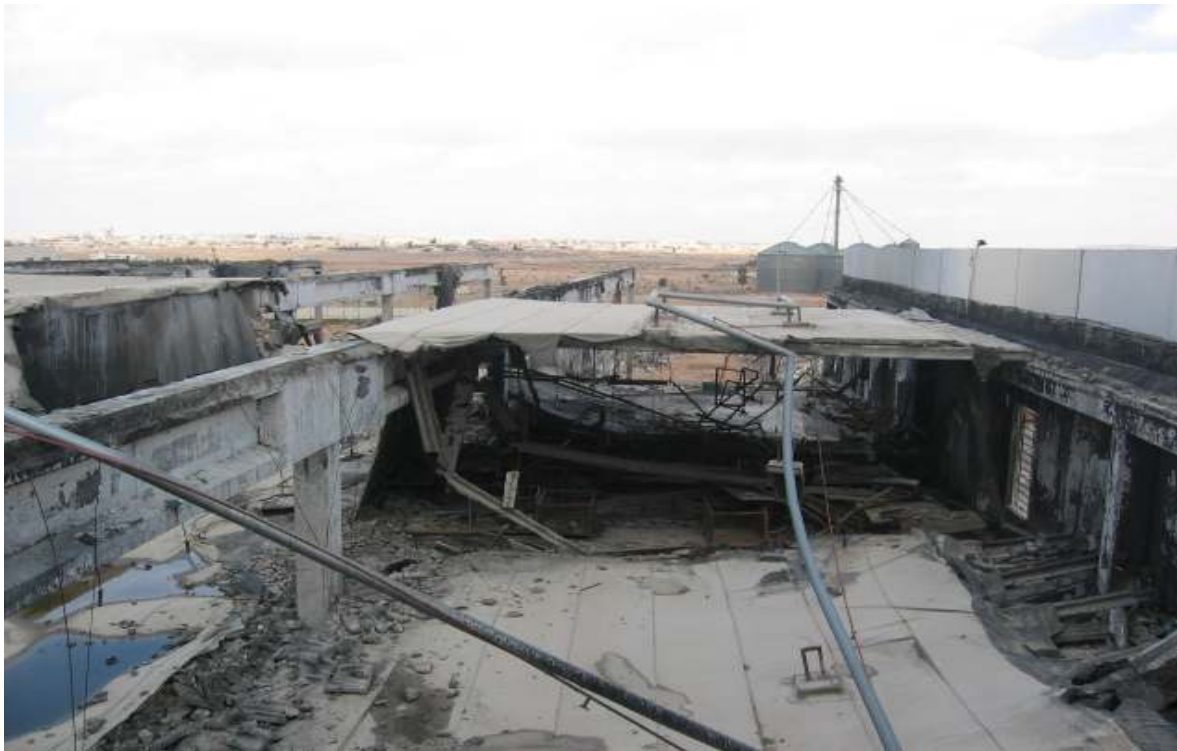
Figure 4 Collapse of slab panels of 1 st floor on ground floor slabs in Zone 2
