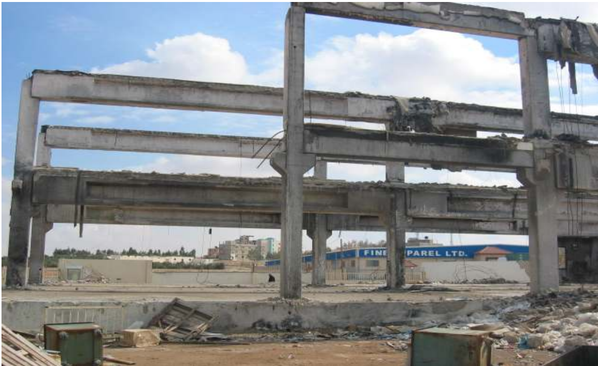
Figure 2 Collapse of slab panels of 1 st and ground floors in Zone 1
