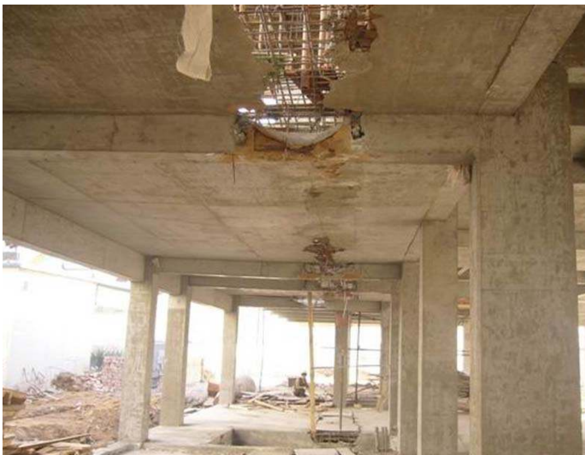
Figure 1 A pour gap problem associated with quality control [6]
