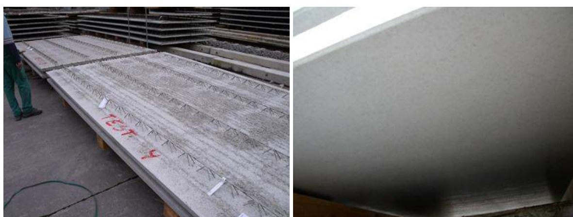
Figure 9 Fabrication of semi-finished slabs with cement reduced ECO-Concrete1 (left), finished surface, view from the bottom (right)
