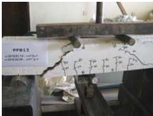
Figure 20 mode of failure PFB12
