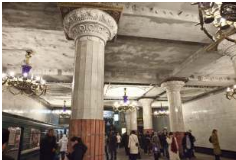
Figure 8 The platform hall of station with the dismantled designs and false ceiling
