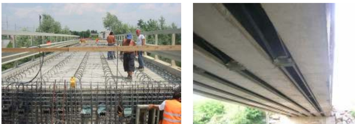
Figure 4 a) Building of new slab connected to the old deck; b) View of externally prestressing
