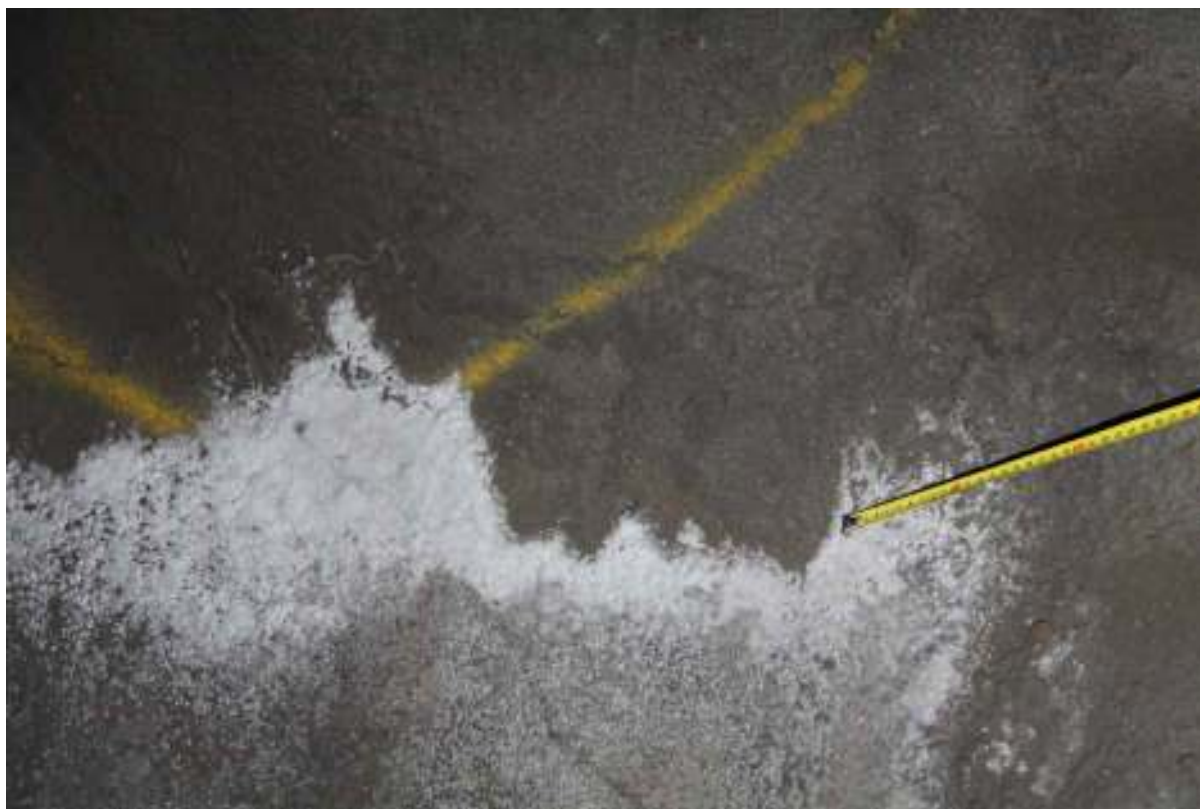
Figure 2 Needle-like efflorescence mirabilite on the concrete surface
