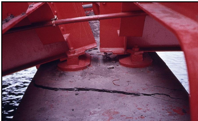
Figure 15: Damage to the shoe of a movable joint of the Showa Bridge, Towhata (1999)
