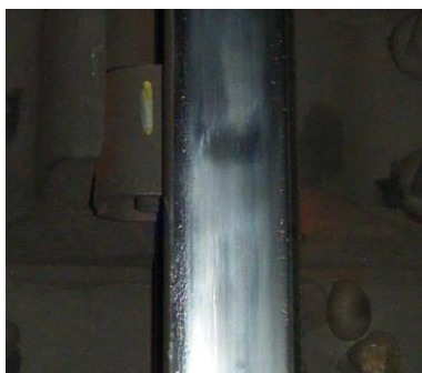
Figure 3: Example of a squat defect observed on the LUL tracks
