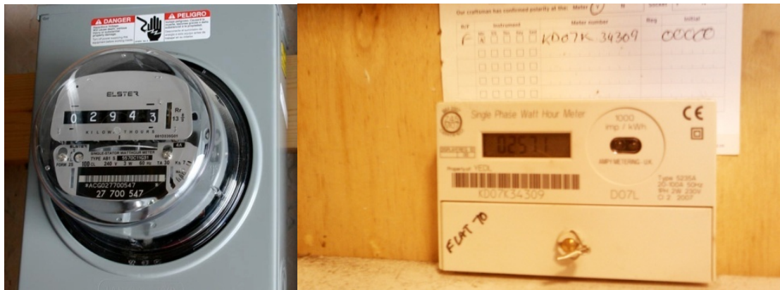
Figure 2.2-3: Household meters, older analogue meter on left, digital meter on right.
