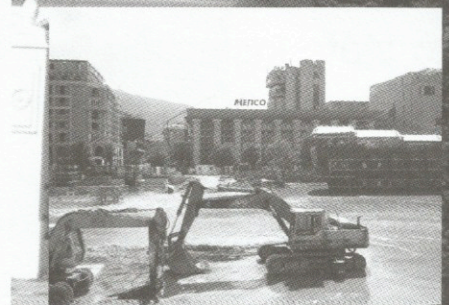
Fig. 11: View of the Headquarters of the Electricity Transmission System Operator of Macedonia (MEPSO) and the construction activities in the riverbed of Vardar in 2016
