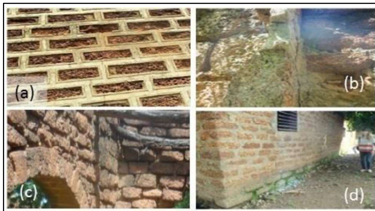
Fig. 4: Views of the most usual defects observed in LDS structures.
