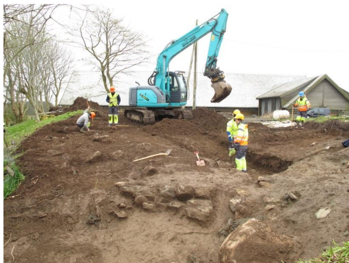
Figure 5.4. Photo of the mechanical topsoil stripping of Area 6, Avaldsnes. Taken facing south, with the flank of Kjellerhaugen, the Bronze Age burial mound, sloping up in the far right foreground of the picture. The boulders visible in the centre for- and middle-ground are from what has been interpreted as a revetment or fortification. Photo: RMP, MCH, UiO.
