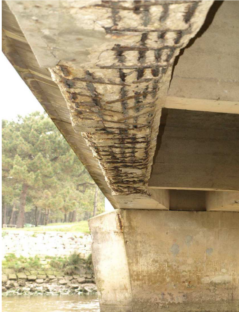
Figure 5: Exposed reinforcement on Girder 1.
