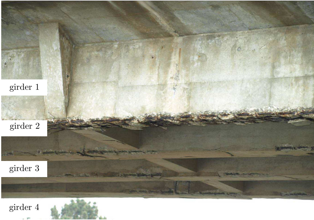
Figure 4: Corrosion affecting girders 1 to 4.
