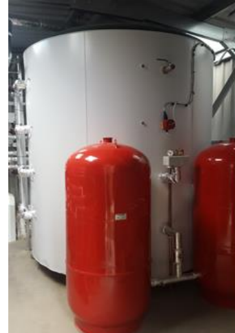
Figure 3 - SCENIC project central thermal store. 10,000 l GALÚ
