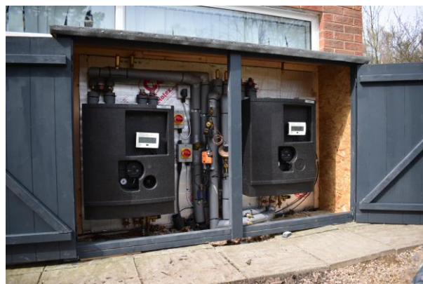
Figure 5 - HIU in situ outside the Tarmac CdFH 4 house. Prosumer unit (right), consumer unit (left)
