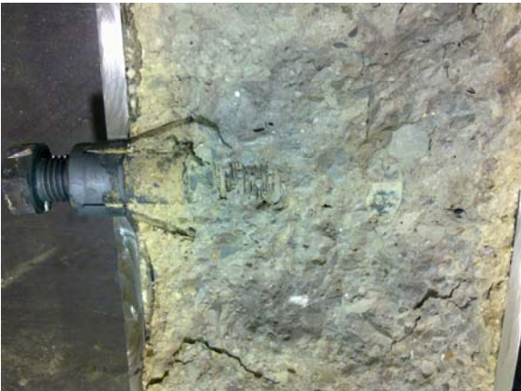
Fig. 9. Specimen after fire exposure.
