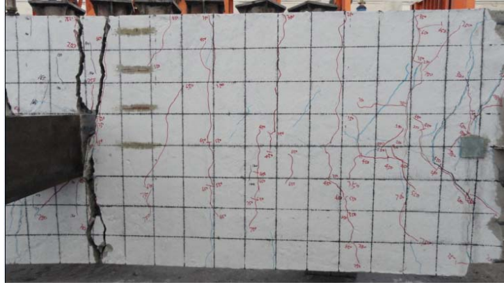
(b)Cracking pattern at top of slab
