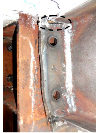
(b)Fracture of welding seam
