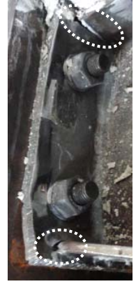
(c)Fracture of welding seam
