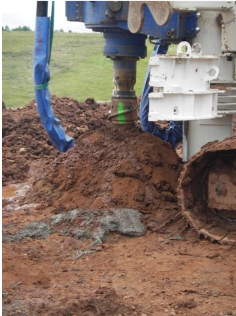
Figure 4.5 The spoil heap produced during installation of pile MR3 and shows a red soup overlying a fine red powder
