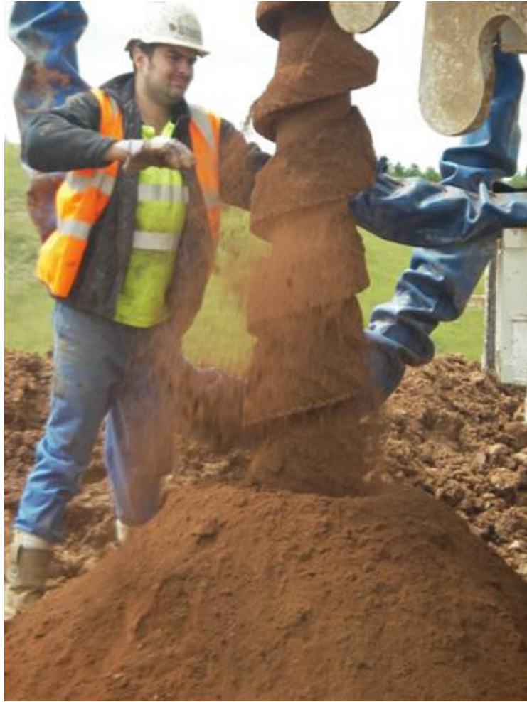
Figure 4.4 The spoil heap produced by the installation of MR2. The spoil heap was a fine powder with some material sticking to the flights of the auger.
