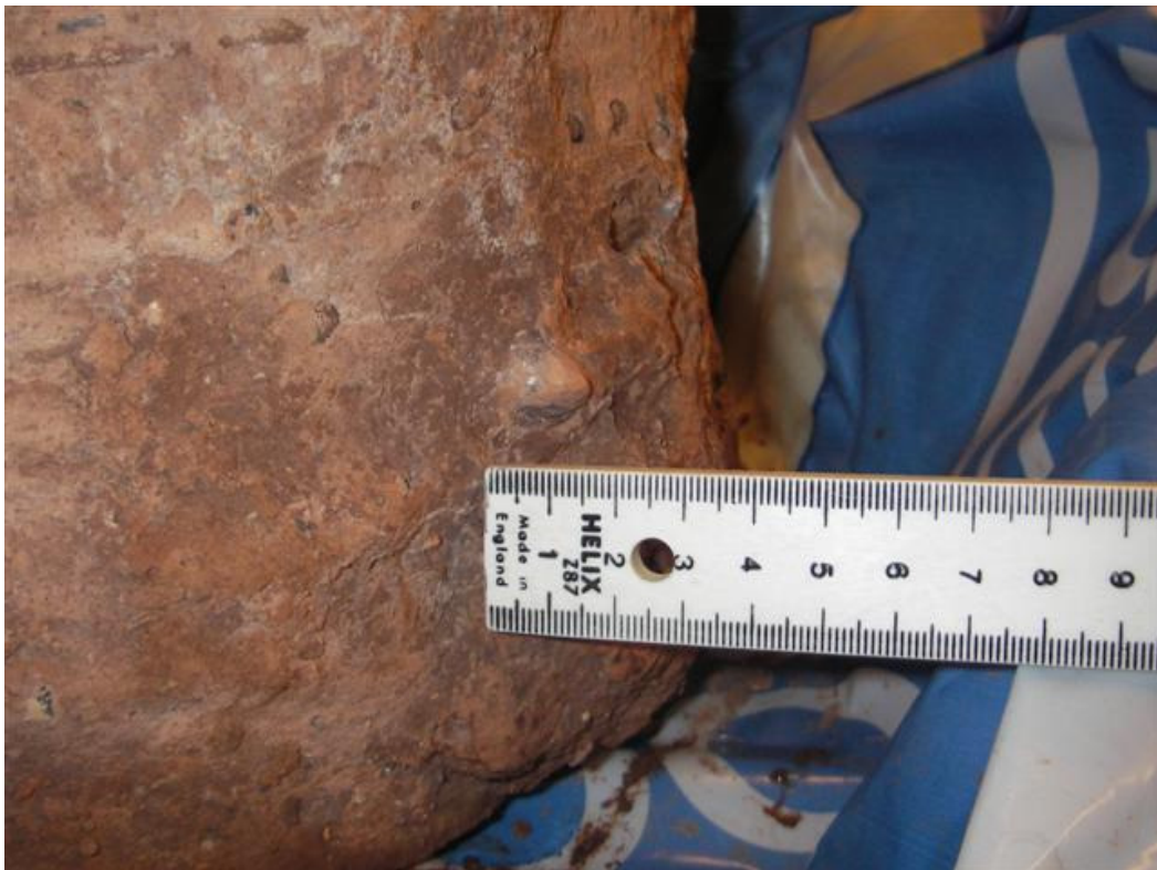
Figure 4.15 Aggregates from concrete of the pile coming out from the surface of the pile shaft. Pile MR1, 0-495mm below ground level.
