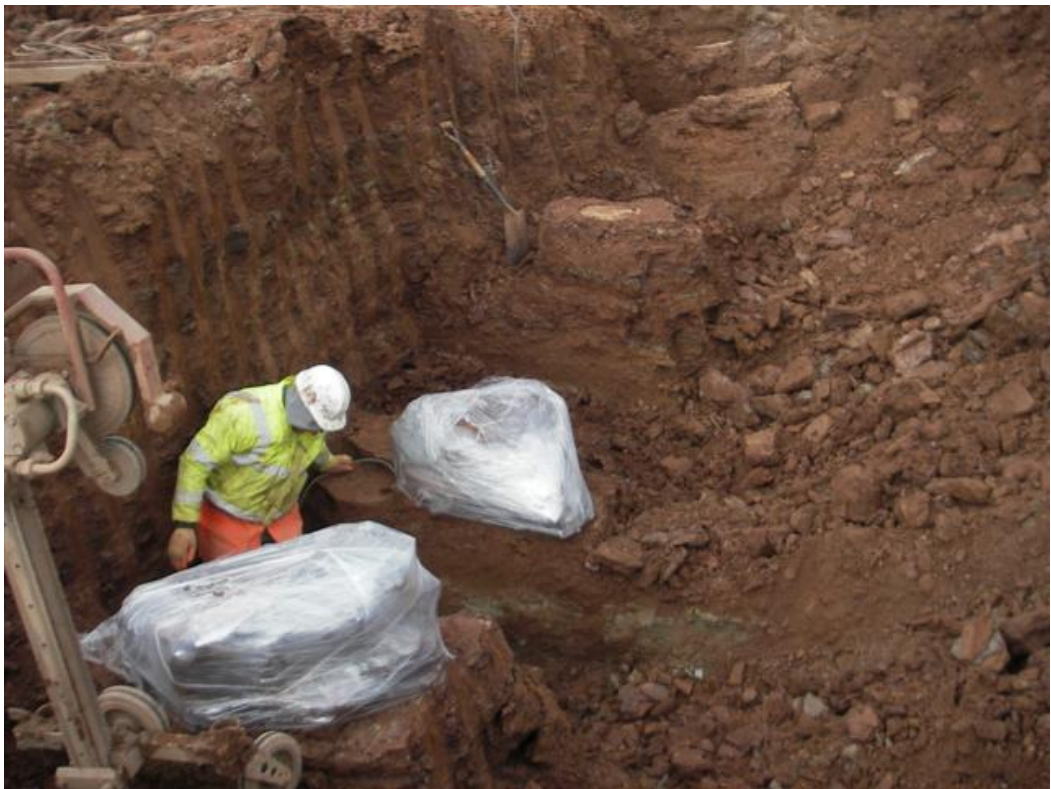
Figure 3.8 Four piles and the surrounding soil, with 2 piles covered in stretchwrap and ready to be cut using the diamond saw
