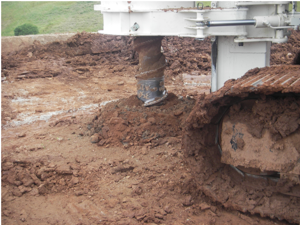
Figure 4.2 Risings during augering of pile MR1 and shows sharp angular blocks of hard material mixed with fine, red/brown powder, as seen while the auger was screwing into the soil
