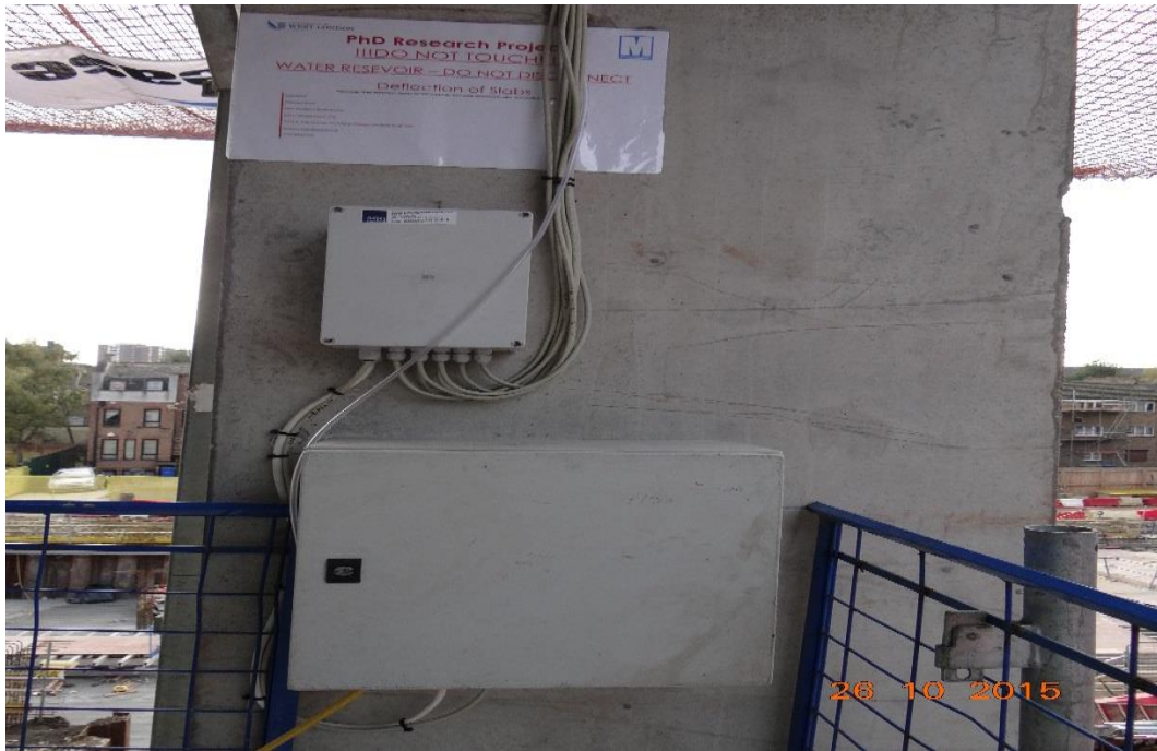
Figure 3.6 Hydraulic Cell Level data box
