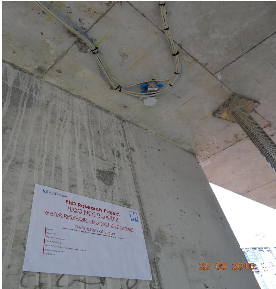
Figure 3.5 Hydrostatic Cell Levelling Location
