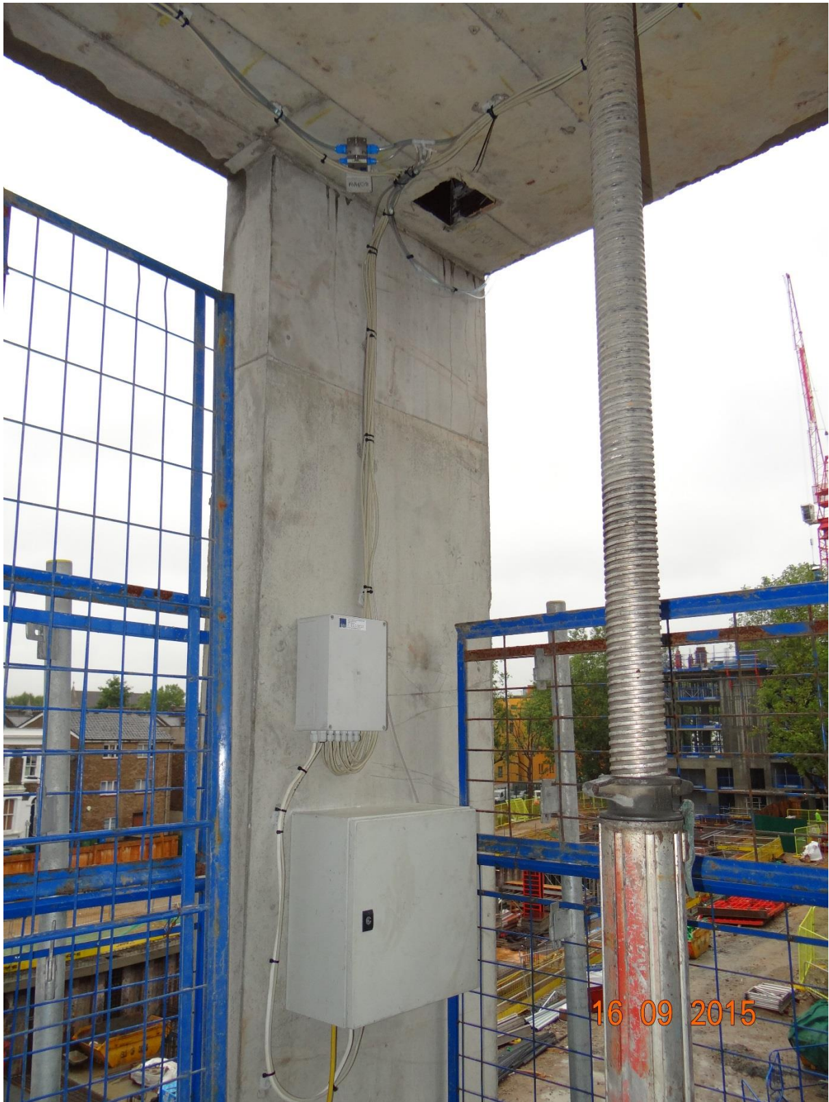
Figure 3.9 Hydrostatic Cells Levelling Connected to Data Box
