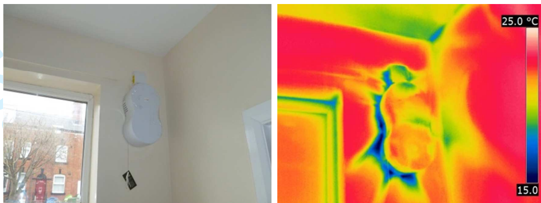
Figure 8 Inadequate sealing of penetrations (extract fan) through IWI seen during depressurisation
