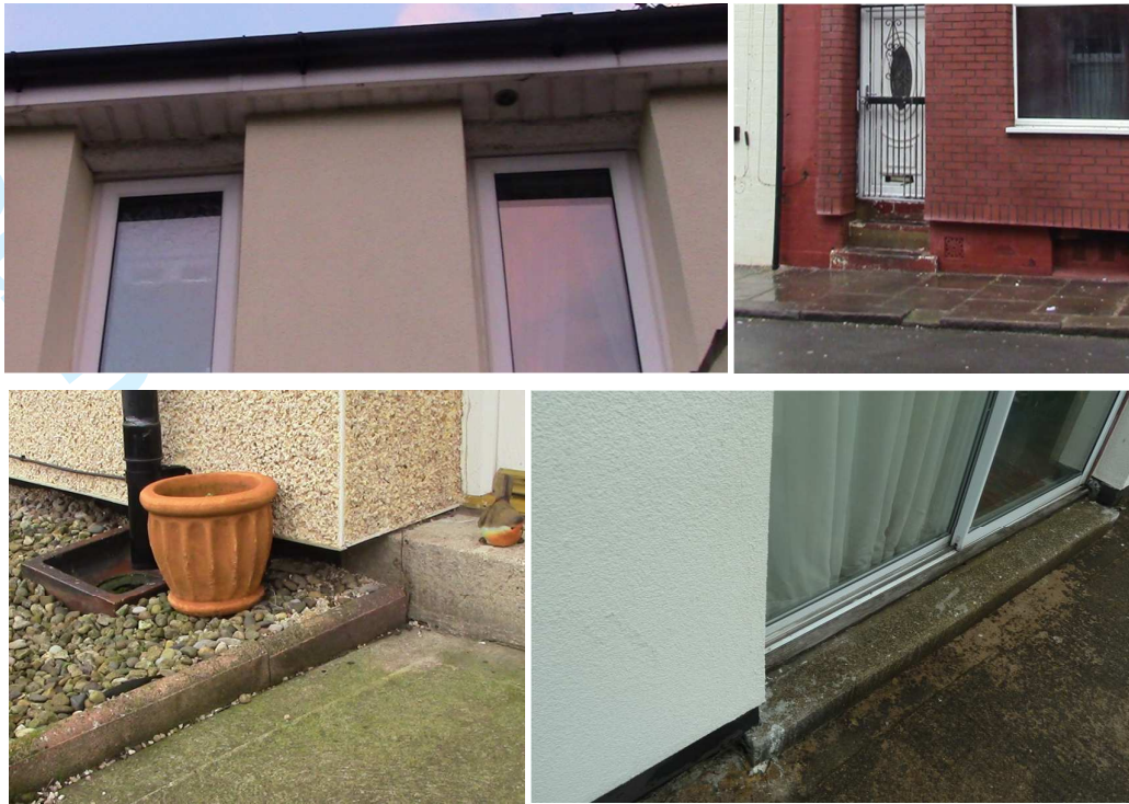
Figure 12 Common EWI details causing thermal bridging
