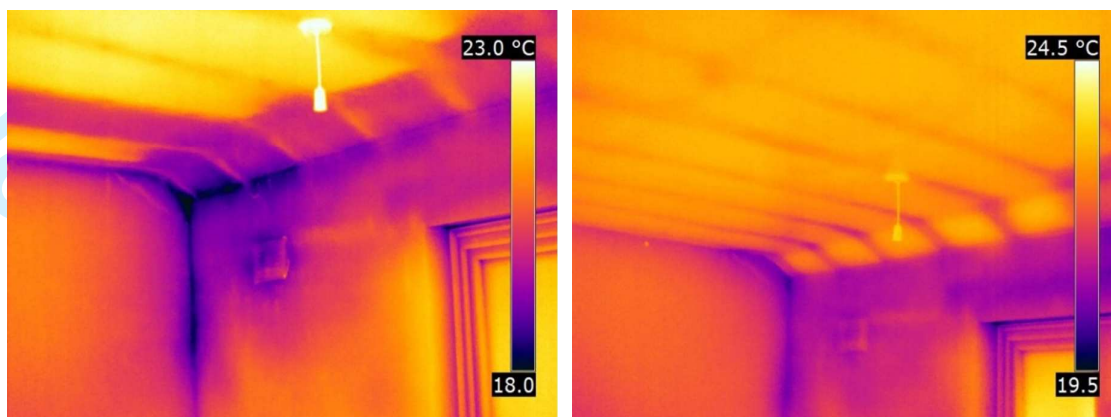
Figure 7 Raked eaves without (left) and with (right) mineral wool cavity batt inserted
