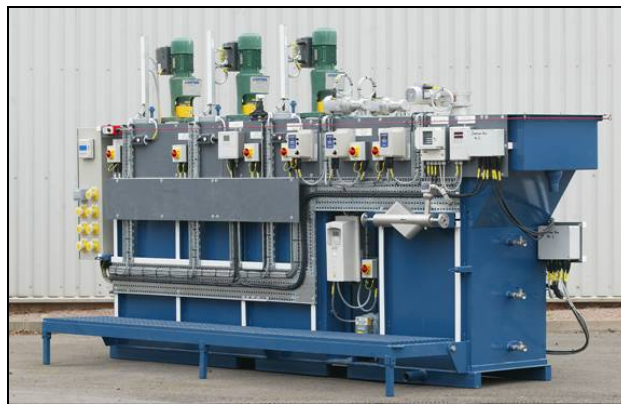
Figure 6. Mynydd Parys pilot active treatment plant.
