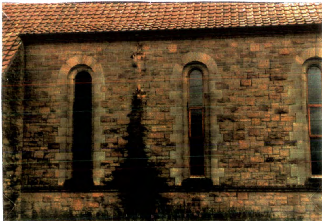
(20) The new hardwood windows (centre and right) do not quite fit in with their stone surroundings as did the one on the left (before it was barred)
