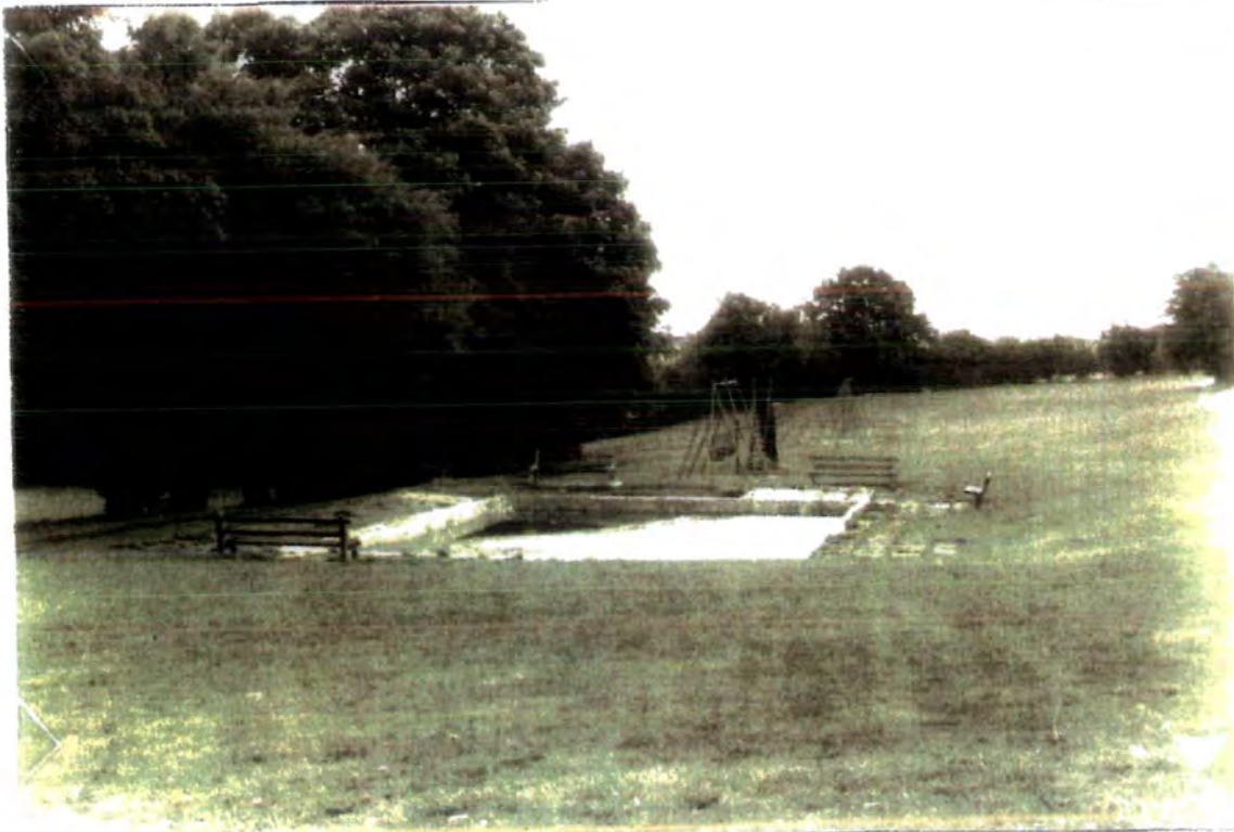
(33) Leisure is the basis of economic regeneration in the Wear Valley. Often older forms of leisure provision are not replaced by the new but left to decay at their side. This childrens' lido has been derelict since before 1982
