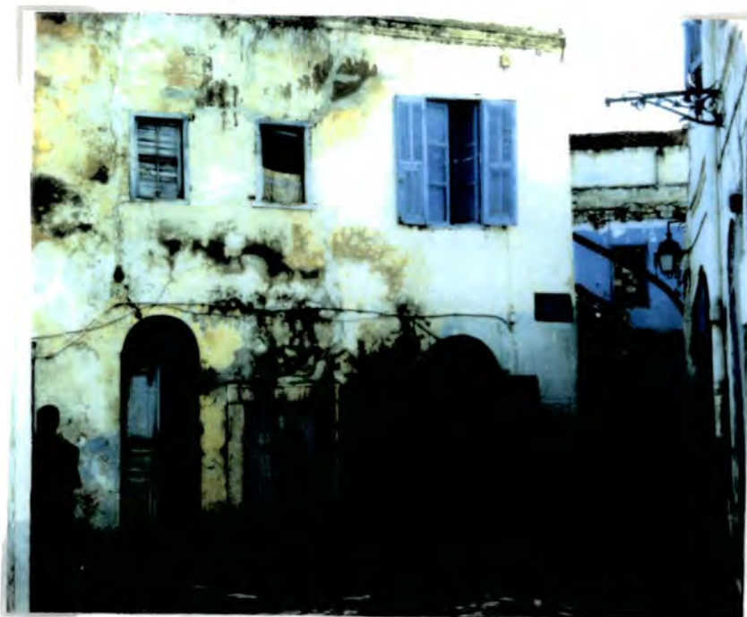
Plate 31: The Oukala (Multi Occupancy) housing problem. Outside view of a decaying oukala on the Rue des Limonadiers. Ownership problems seemed to be at the heart of the problem for this building. In January 1991 the building was recommended for demolition.
