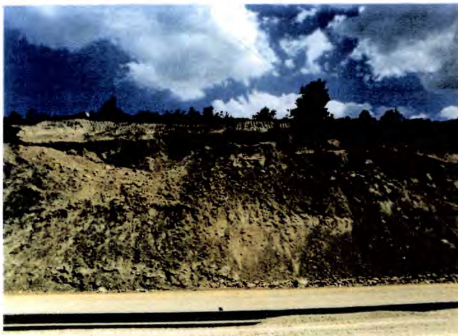
Photograph 3.2 Slope failure at position ARV3
