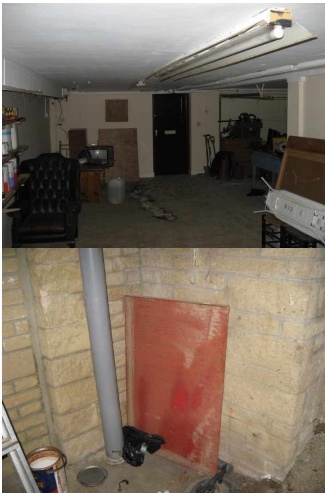
Figure 5.3: Two adaptations to flooding at a house in Helmsley. Top: the lower floor of the house, not used as a living space and largely cleared out of valuables. Bottom: a wooden barricade.
