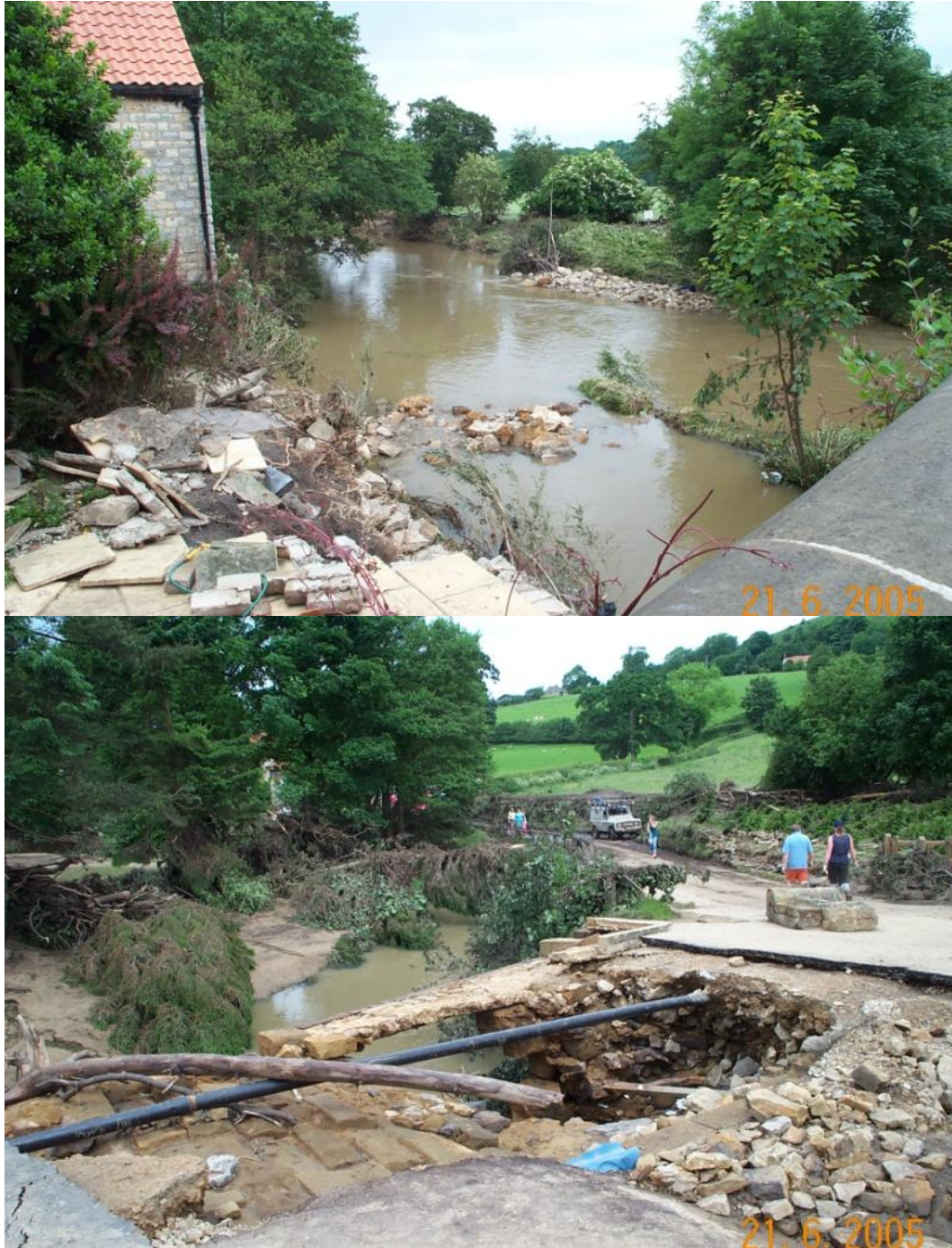
Figure 1.5: Damage caused by the 2005 flash flood event in upper Ryedale, photographs taken at Helmsley (top) and Hawaby (bottom), showing damage to infrastructure and property in addition to the deposition of large amounts of fine sediment and debris. Photographs provided by Jeff Warburton.
