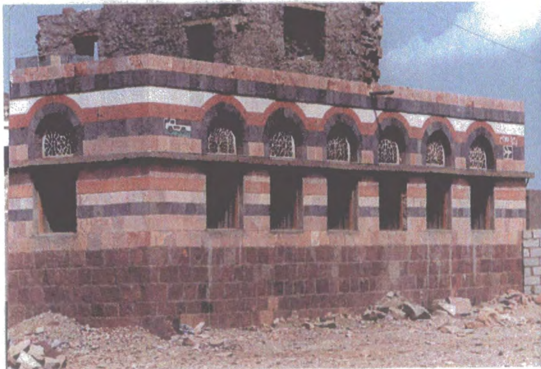
Top left - Repairing of cracks associated with random decorative effects, Sana'a; right - Sana'a. The covered roof terrace suggests a tenant from the Tihama. Notice model of Sana'ni house at the roof corner; centre left - Dhamar; right - Rada'; bottom - Jubban; opposite, top left - Jubban; right - Hajja; centre, left - Hayma; right - Al Dahi; bottom - Hajja
