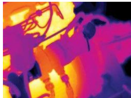
Figure 23: Thermal image of pump (Source: FLIR Systems, Inc.)
