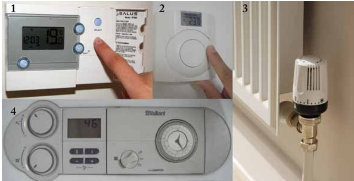
Figure 1.2 Examples of Heating Controls (clockwise from top left: 1-programmable thermostat, 2-manual room thermostat, 3-thermostatic radiator valve on a radiator and 4-boiler interface with manual programmer)
