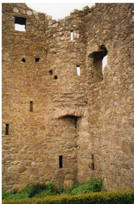
Figure 97. Tully Castle. Illustrating corbelled out stair turret from the first to second floor. Photographer: C. Ryder.
