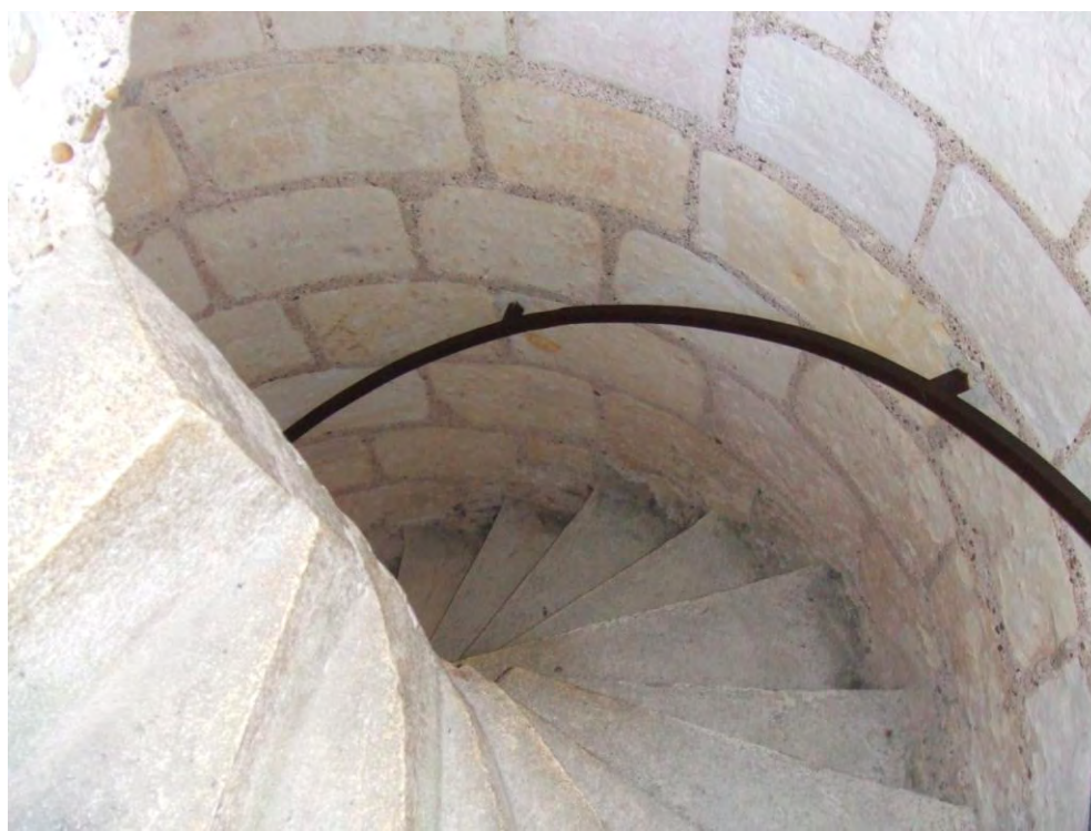
Figure 37. Loches: Interior Spiral Stair. View of the spiral stair leading to the elite accommodation in the grosse tour . Photographer: C. Ryder.
