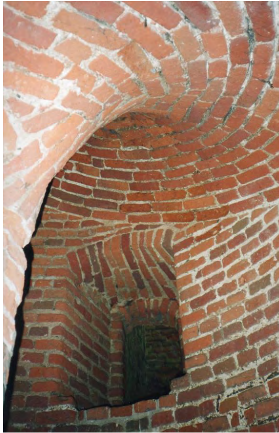
Figure 100. Kirby Muxloe: Brick Spiral Stair. Illustrating brick vaulting supporting the brick spiral stair. Photographer: C. Ryder.
