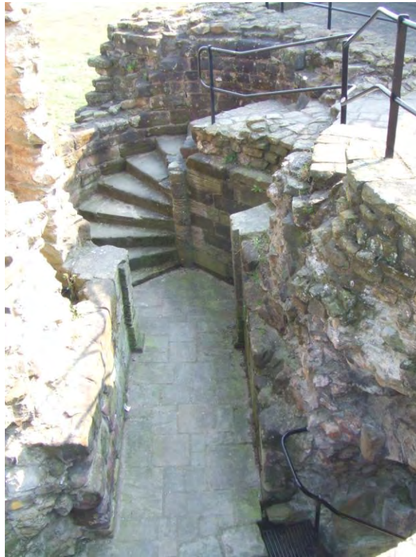
Figure 69. Flint Castle Donjon. Illustrating spiral stair in the Donjon to the upper floors. Photographer: C. Ryder
