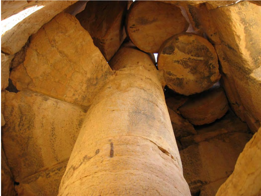
Figure 35. Palmyra, Temple of Bel: Spiral Stair. Illustrating structure of the spiral stair from below. http://publicimages.org/freeimage/ViewImage.aspx?imageId=3918032 .
