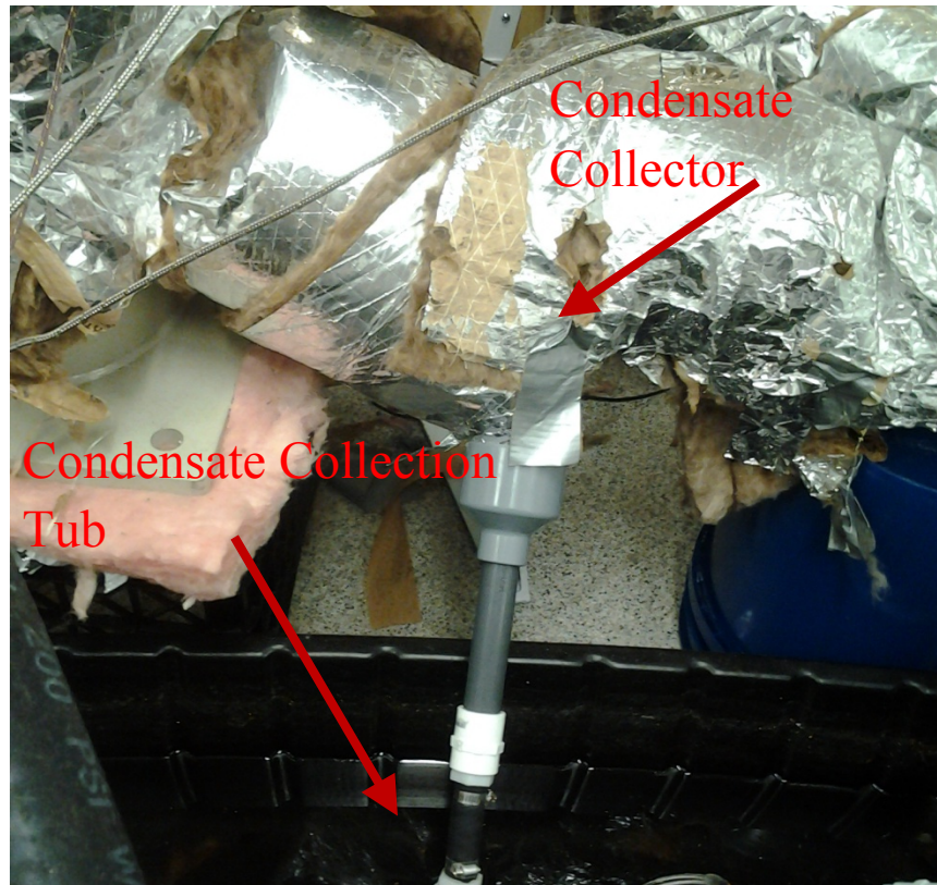
Figure 3-15: Condensate collector angled downward towards tub
