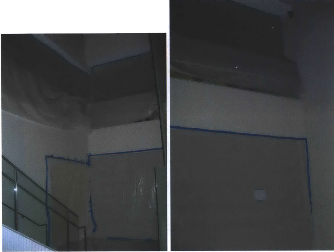
Figure 5-5: Mounted polyethylene 4 mm flame retardant tarp used to seal various openings to atrium. The NE opening on the first and second floor (left) and SE opening on the first and second floor (right) are shown.
