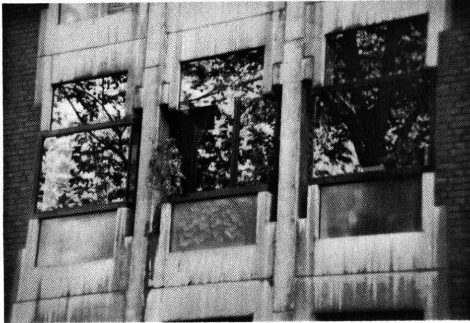
Detail view of precast concrete structural pieces, apartment/office building in Amsterdam by Abel Cahan.
