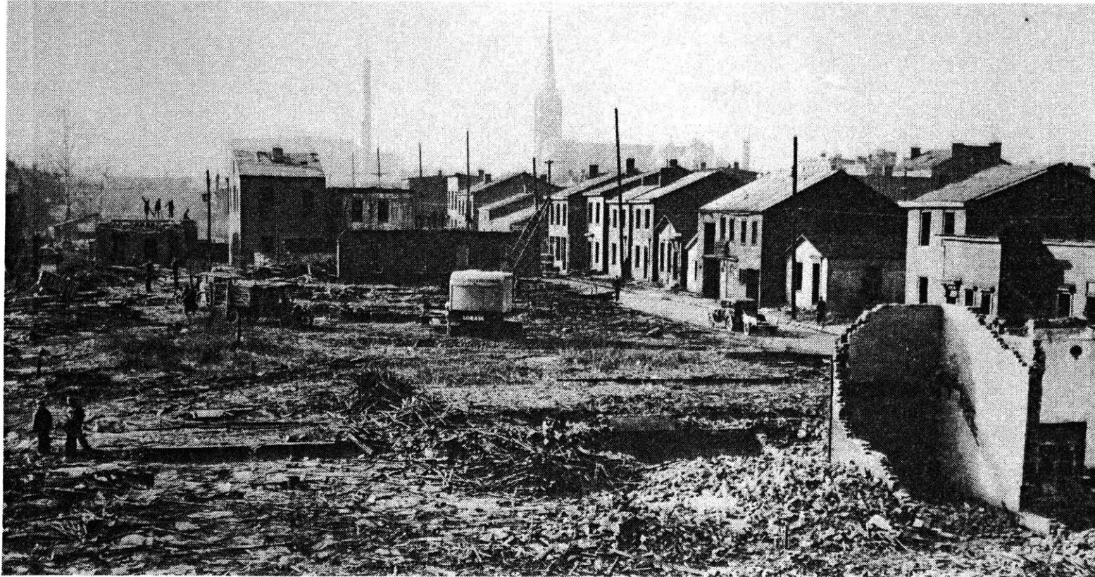
Wrecking operations, south of Marshall. St. Boniface Church is in the background.
