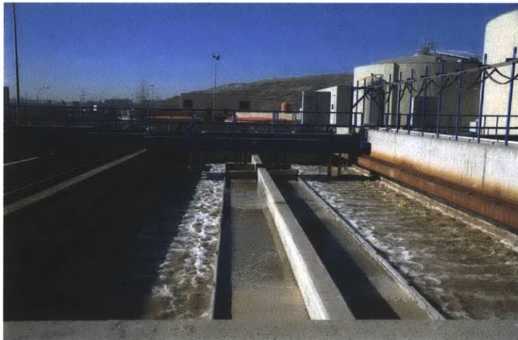
Figure 2.11 Aerated Grit Chamber
