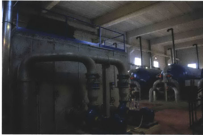
Figure 2.13 Tertiary Treatment: Filtration Tanks and UV Disinfection
