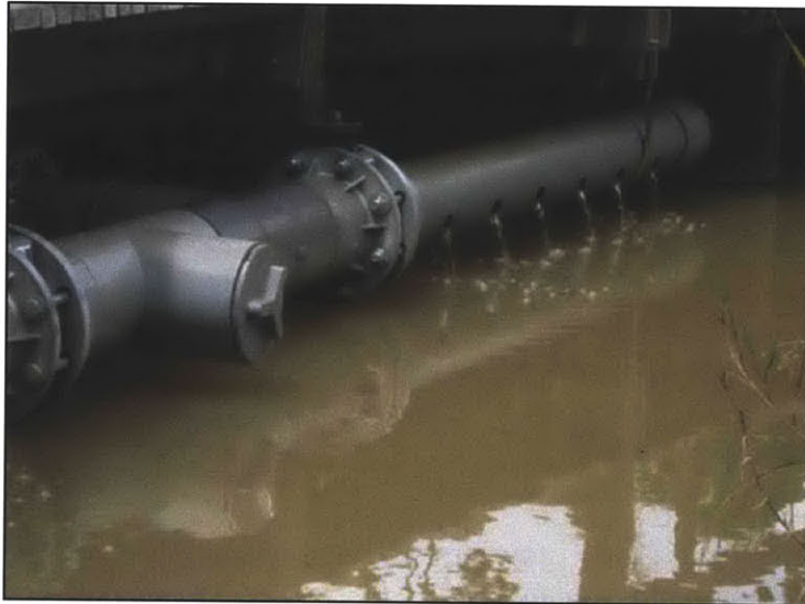
Figure 18 - Inlet of wetland systems
