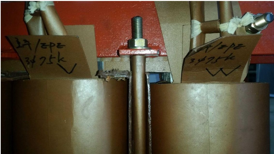
Figure 6.45 – Close north facing view of the top outer C windings core leg (bulk windings movement) – 100% axial shift to the bottom of the core window.
