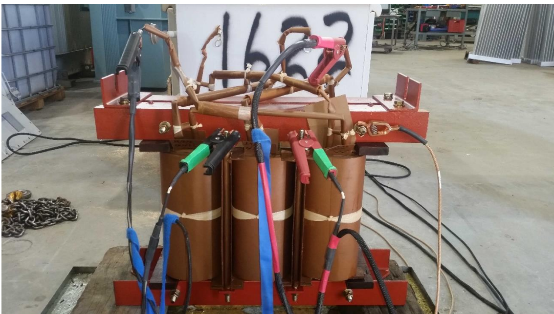
Figure 6.28 - Un-tanked (New Benchmark) open circuit SFRA test set connection
