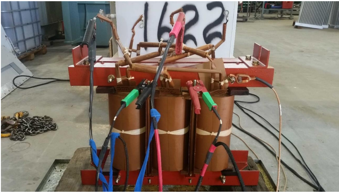
Figure 6.27 - Un-tanked (New Benchmark) open circuit SFRA test set connection
