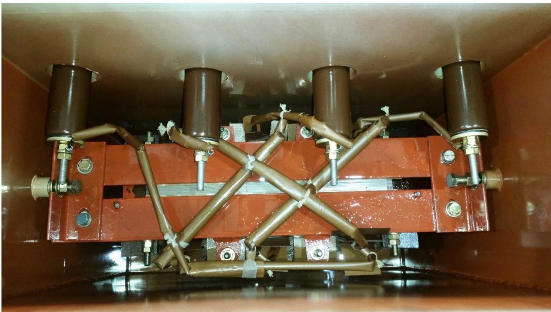
Figure 6.14 - Photo of the test earthing transformer internals with the lid removed and oil removed.
