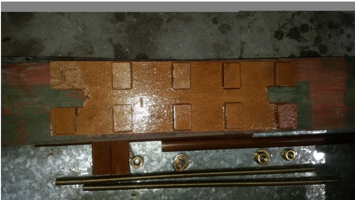
Figure 6.41 – Inter-winding insulation packer once removed, prior to modification
