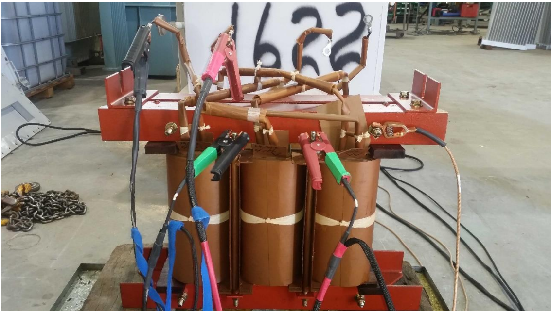
Figure 6.26 – Un-tanked (New Benchmark) open circuit SFRA test set connection
