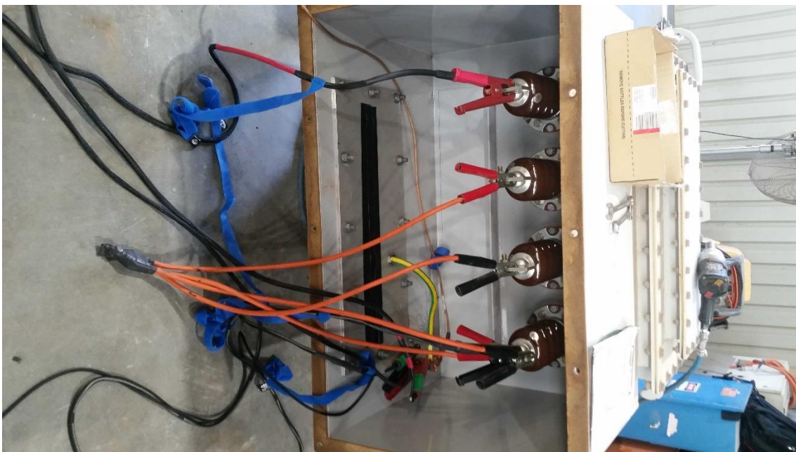
Figure 6.11 - Short circuit SFRA test set connection
