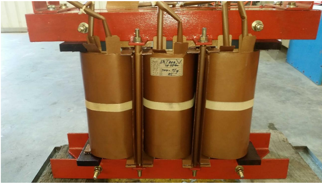
Figure 6.23 – South side photo of the test earthing transformers core and coils sitting on top of two large wooden blocks in a metal oil containment tray.
