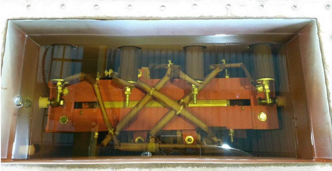
Figure 6.13 – Photo of the test earthing transformer internals with the lid removed and full of oil.
