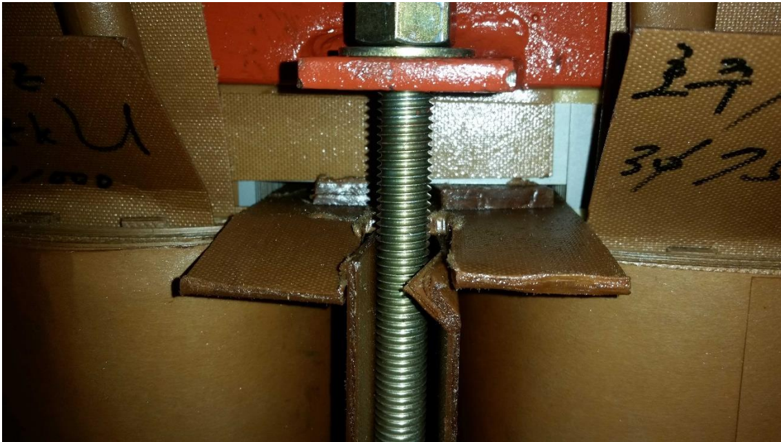
Figure 6.38 – Close photo of the inter-winding insulation packer prior to removal.
