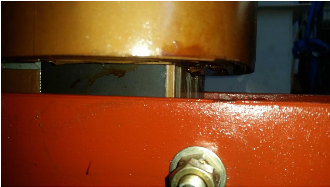
Figure 6.48 - Close north-east facing view of the bottom outer C windings core leg (bulk windings movement) – 100% axial shift to the bottom of the core window.
