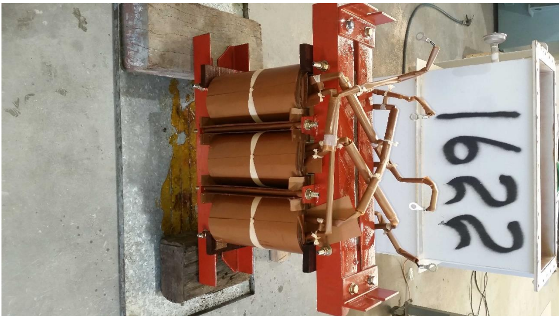
Figure 6.22 – North side photo of the test earthing transformers core and coils sitting on top of two large wooden blocks in a metal oil containment tray with connection leads visible.
