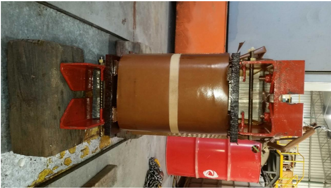
Figure 6.25 - East side photo of the test earthing transformers core and coils sitting on top of two large wooden blocks in a metal oil containment tray.
