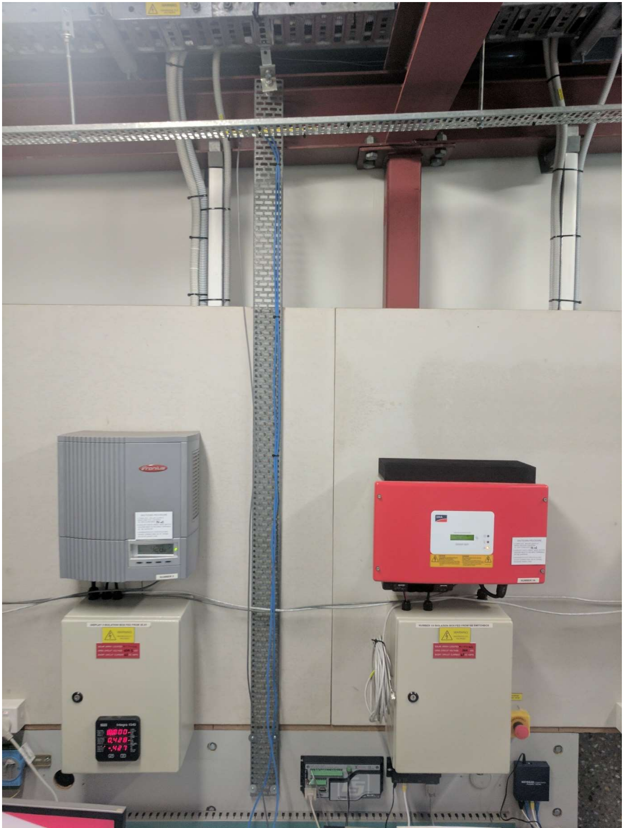
Figure 14 Cable Tray Housing Data Cables in Level 3 EEB
