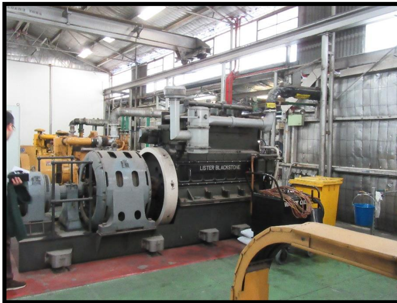
Figure 29 Detroit Generator at Rottnest Island Power Station
