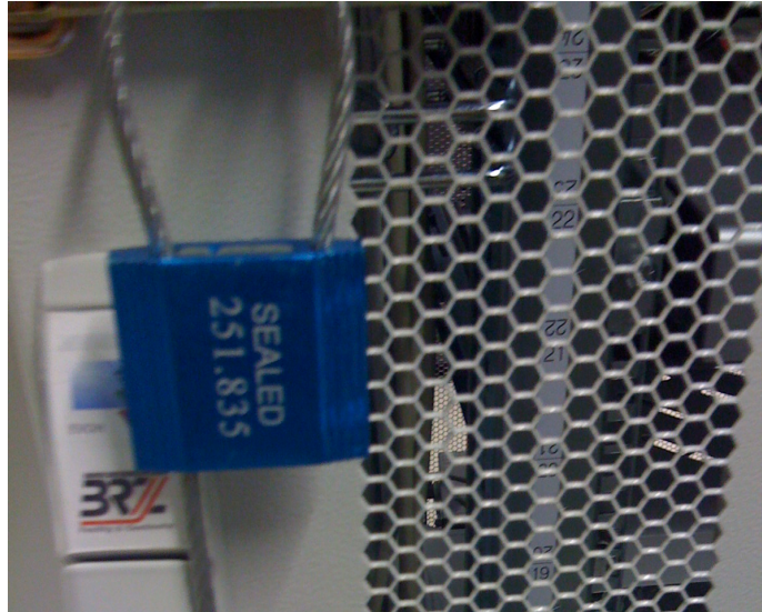
Figure 38: Sealed protective Cabinet
