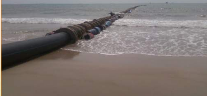
Marine outfall pipeline (sea portion)
