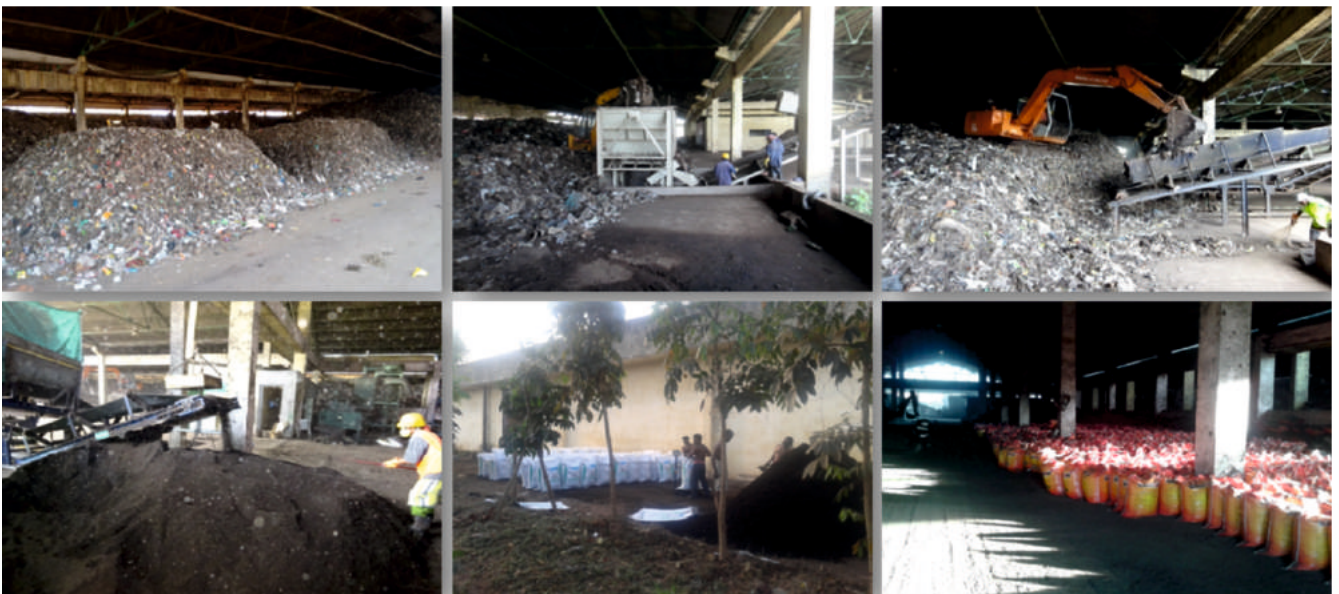
Windrows at Processing Yard, uploading waste through hopper, Sieving through 4mm, city compost Bagging
