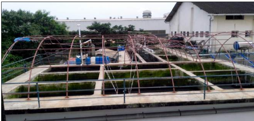
Effluent Treatment Plant
