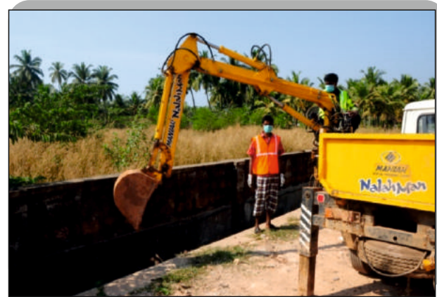
Figure 4 Drain Cleaning machine
