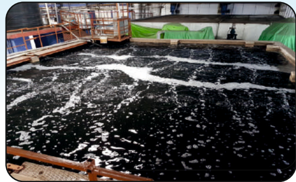
Effluent treatment plant
