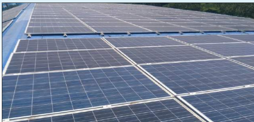
Solar Panels established on the cold storage roof top
