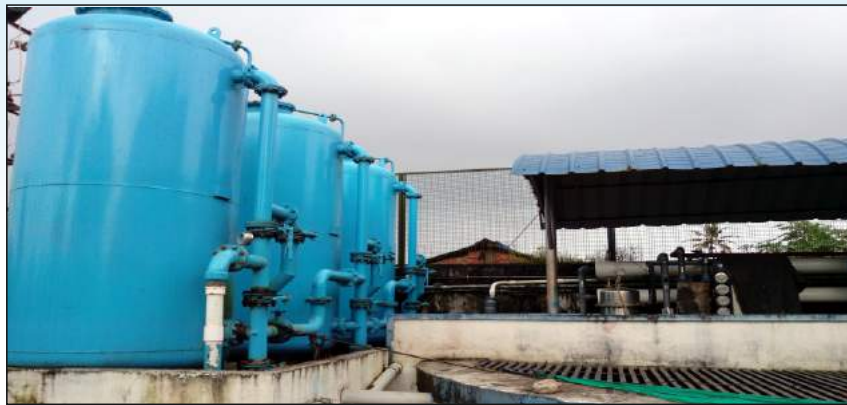
Water Treatment Plant (RO)
