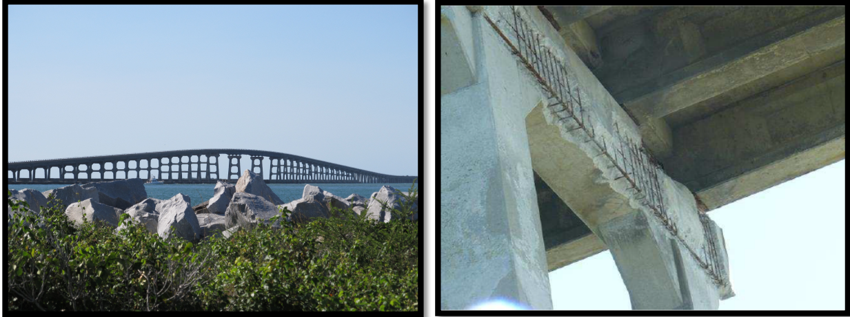
Figure 5.1: Left – Bonner Bridge, 2012 (Photo by D Swain); Right – Structural Deterioration to Bridge, 2008 (OBTF 2008)
