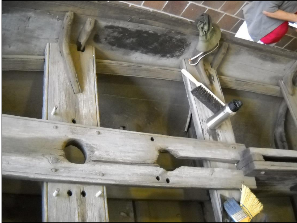
Figure 35: Forward Mast Partner and Supporting Structures from Port Side (photo by ECU Fall Field School 2010)
