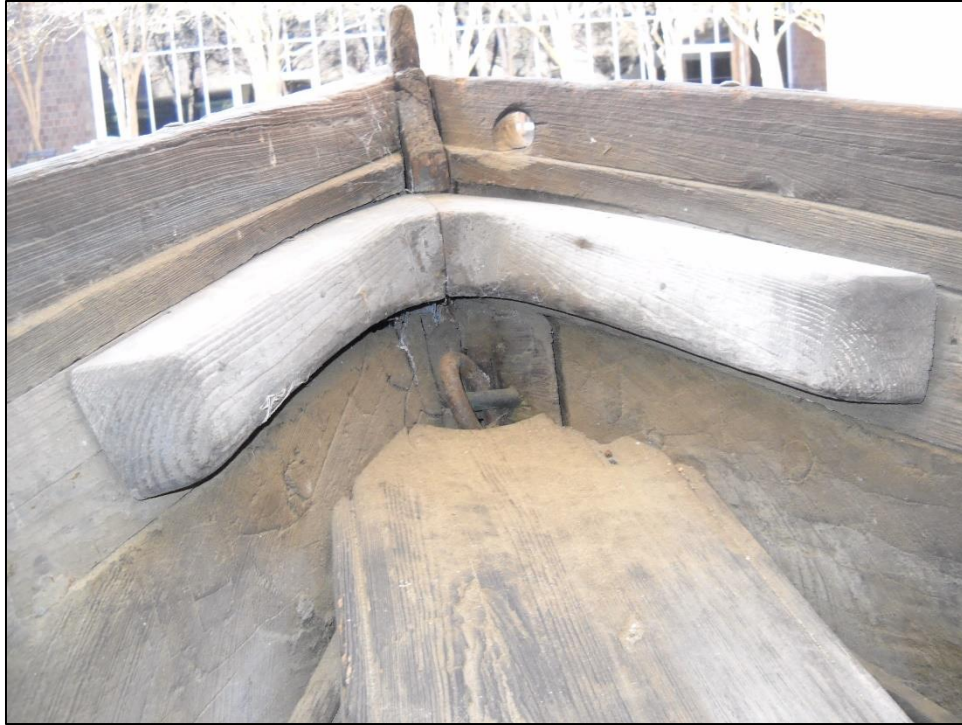
Figure 33: Close Up of Interior Bow and Breasthook from above the Mast Partner (photo by ECU Fall Field School 2010)
