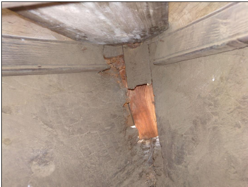
Figure 34: Close Up of Interior Bow and Repairs from below the Mast Partner (photo by author 2012)
