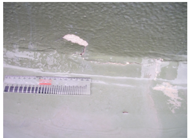
Figure 6: WATERPROOF MEMBRANE CRACKING
