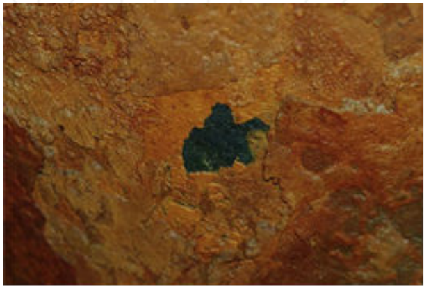
Figure 1. Accelerated Low Water Corrosion Observed on Steel Piles above Water during Spring Tide [2]
