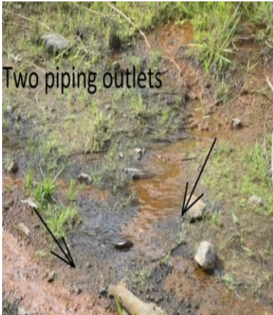
Figure1 Piping outlets leading to seepage
