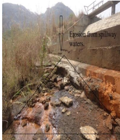
Figure10 Scouring at dam toe
