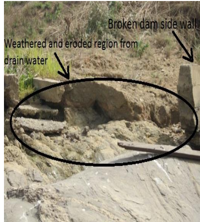
Figure 2 Broken and Eroded part of drainage at right-side retaining wall
