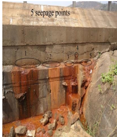
Figure 8 Concrete body seepage
