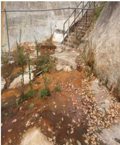
Figure 7 Seepage from the concrete/rock interface
